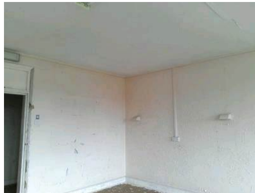
Ref. Sample 31: Building 142. First Floor. 112. Textured coated plasterboard ceiling and associated debris to floor
