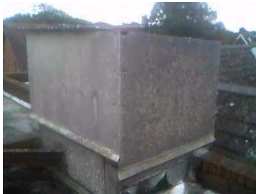
Sample 124: Building 165. External. Flat Roof Area. Cement wall panels by water tank
