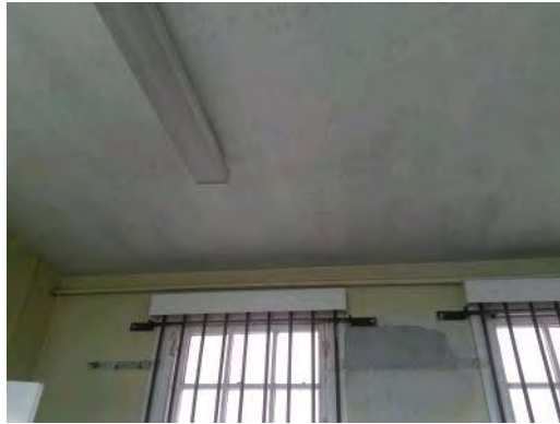
Ref. Sample 2: Building 142. Ground Floor. 002. Textured coated plasterboard ceiling
