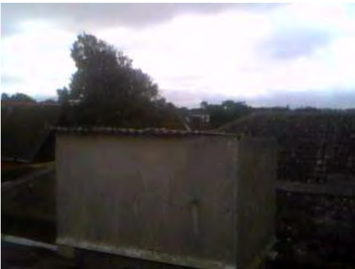
Sample 123: Building 165. External. Flat Roof Area. Corrugated cement roof sheets by water tank
