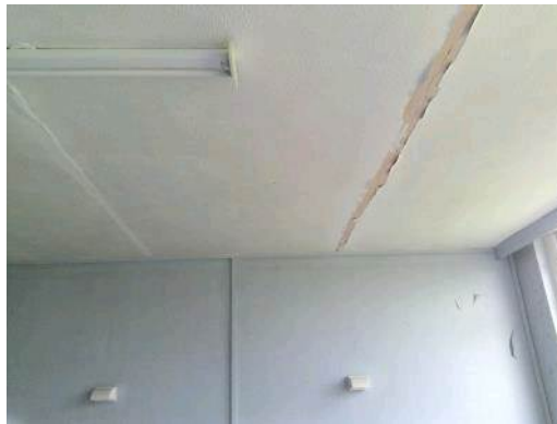
Ref. Sample 19: Building 142. Ground Floor. 018. Textured coated ceiling and associated debris to floor
