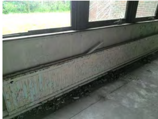
Sample 24: Building 142. Ground Floor. 014. Cement panels under windows around entrance lobby and behind wooden cladding above entrance doors
