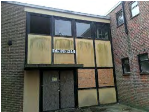
Sample 49: Building 142. External. Externals. Cement panels (painted yellow) above 1st floor windows, and to front and rear of foyer areas
