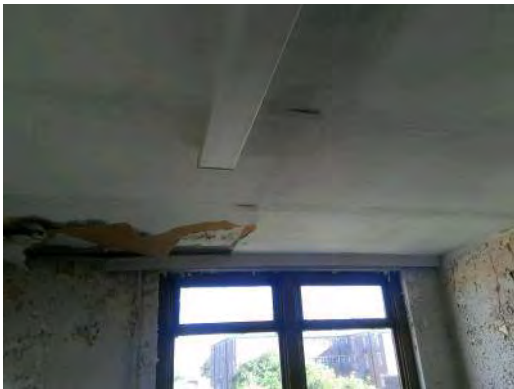
Ref. Sample 36: Building 142. First Floor. 115. Textured coated plasterboard ceiling and associated debris to floor
