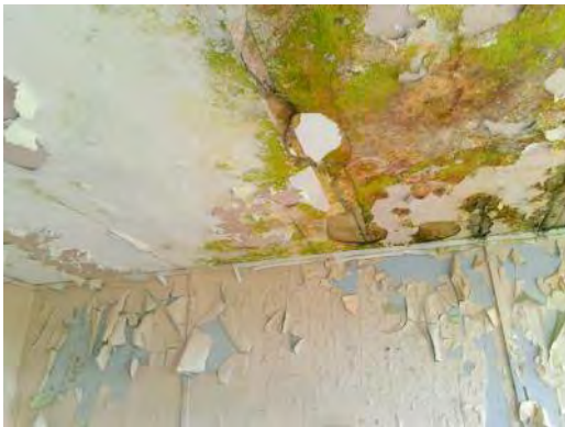
Sample 19: Building 142. Ground Floor. 016. Textured coated ceiling and associated debris to floor
