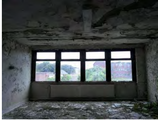
Sample 36: Building 142. First Floor. 113. Textured coated plasterboard ceiling and associated debris to floor
