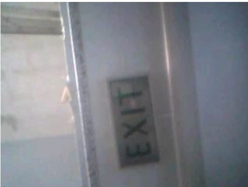
Ref. Sample 66: Building 165. Ground Floor. Stairway 2. Textured coating to ceiling and associated debris to floor
