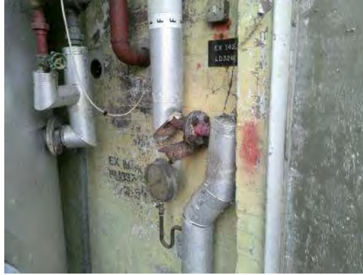
Sample 44: Building 142. Ground Floor. 021. Gaskets to flanges of pipework
