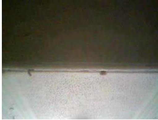
Ref. Sample 72: Building 165. First Floor. Toilets 34. Textured coating to ceiling
