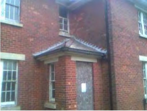
Sample 128: Building 165. External. Main Building. Cement roof tiles and associated debris
