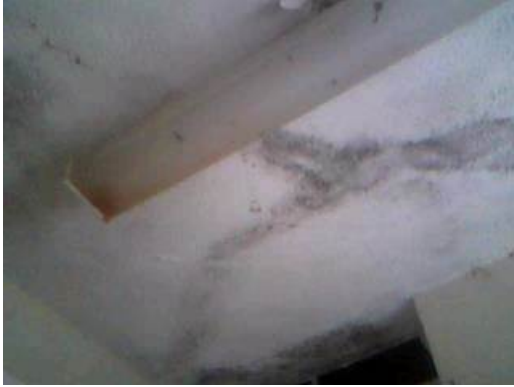
Ref. Sample 96: Building 165. First Floor. Toilets 55. Textured coating to ceiling
