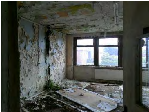
Sample 31: Building 142. First Floor. 110. Textured coated ceiling and associated debris to floor
