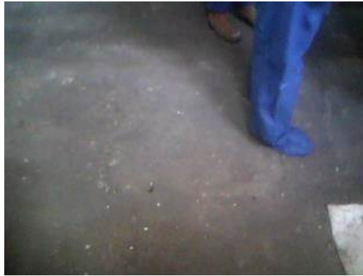
Sample 4: Building 165. Ground Floor. Boiler House. Dust and debris to floor
