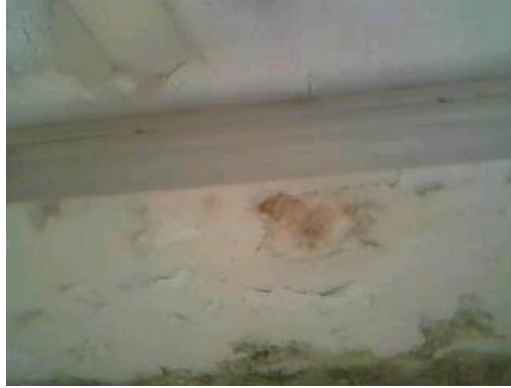
Sample 31: Building 165. Ground Floor. Room 19. Textured coating to ceiling and associated debris to floor
