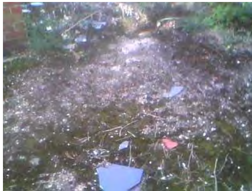
Sample 57: Building 165. External. Courtyard. Cement tile debris to floor throughout
