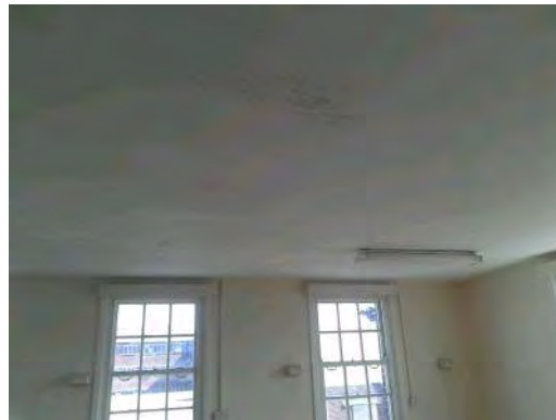
Ref. Sample 26: Building 142. First Floor. 108. Textured coated plasterboard ceilings above stairs and end of corridor
