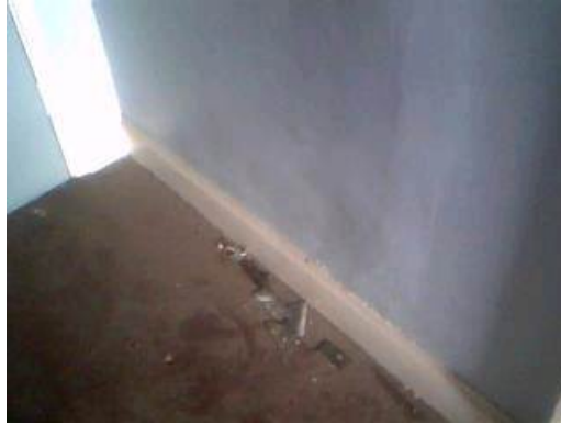
Sample 108: Building 165. First Floor. Corridor 6. Stair nosing debris to floor
