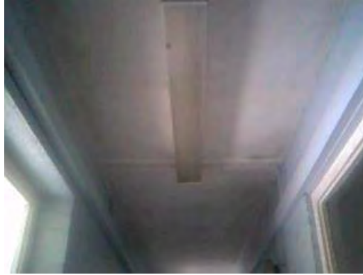
Sample 66: Building 165. Ground Floor. Corridor 2. Textured coating to ceiling and associated debris to floor
