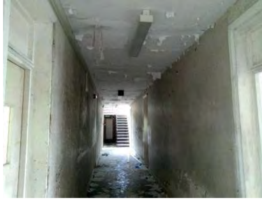
Sample 12: Building 142. Ground Floor. 014. Textured coated ceiling and associated debris to floor
