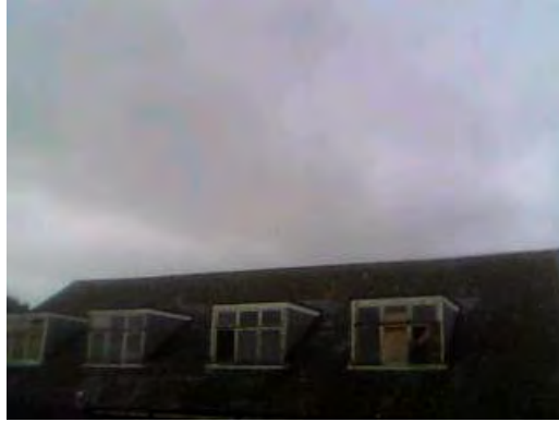
Sample 122: Building 165. External. Flat Roof Area. Cement roof tiles and associated debris
