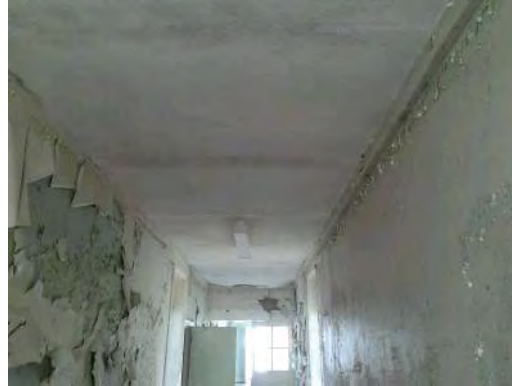
Sample 30: Building 142. First Floor. 109. Textured coated plasterboard/concrete ceiling and associated debris to floor
