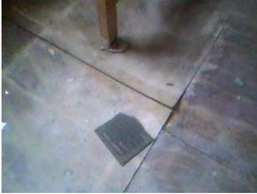
Sample 104: Building 165. First Floor. Room 36. Cement tile debris to floor
