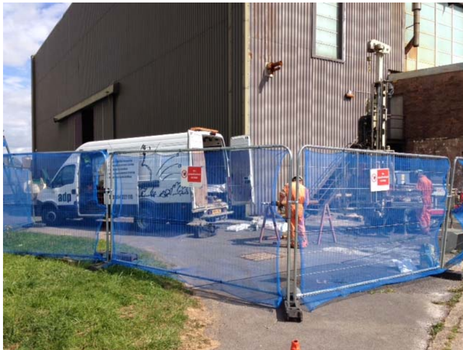
Borehole installation at CELBH03 adjacent to the south west corner of Dunning Hanger
