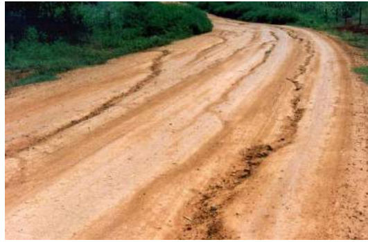
Longitudinal erosion in fine material
