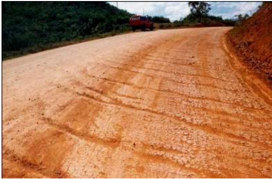
Transverse erosion in fine material
