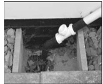
Waste pipe non-return valve
