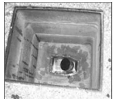
Foul chamber non-return valve
