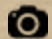
Royal Engineers from 37 (Three Seven) Squadron strip a medium girder bridge (Picture Sgt Wes Calder RLC)
