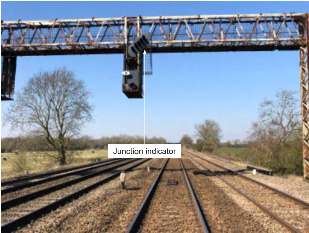
Figure 3: Signal LR507 with position 4 junction indicator (picture courtesy of Network Rail)
