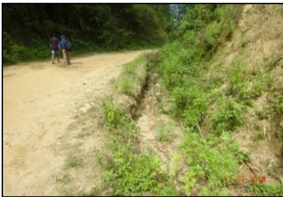
Photo 3: Roadside and drainage damage, July 2017
