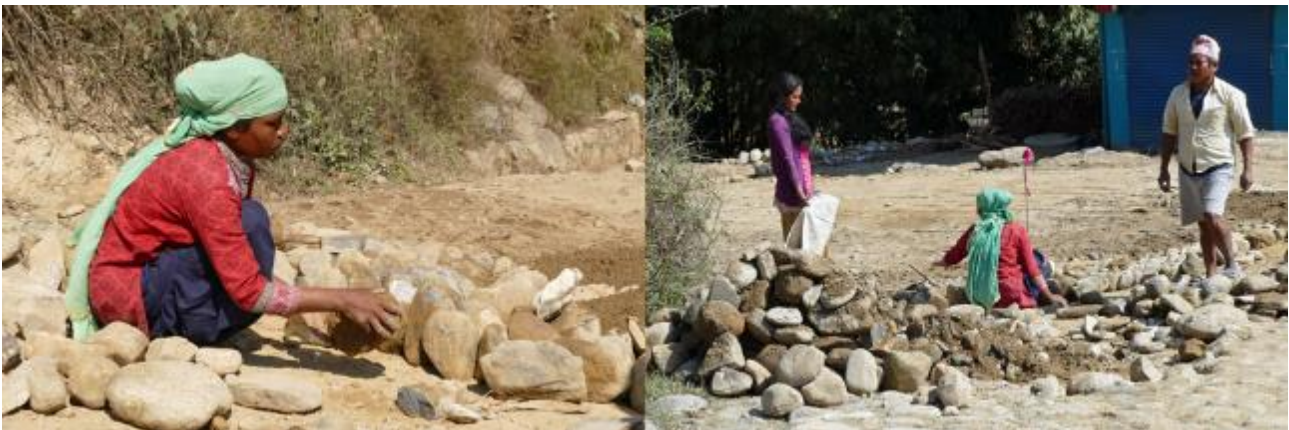
Figure 32 Male and female stone masons and a female labourer repairing a cobblestone section of the road
