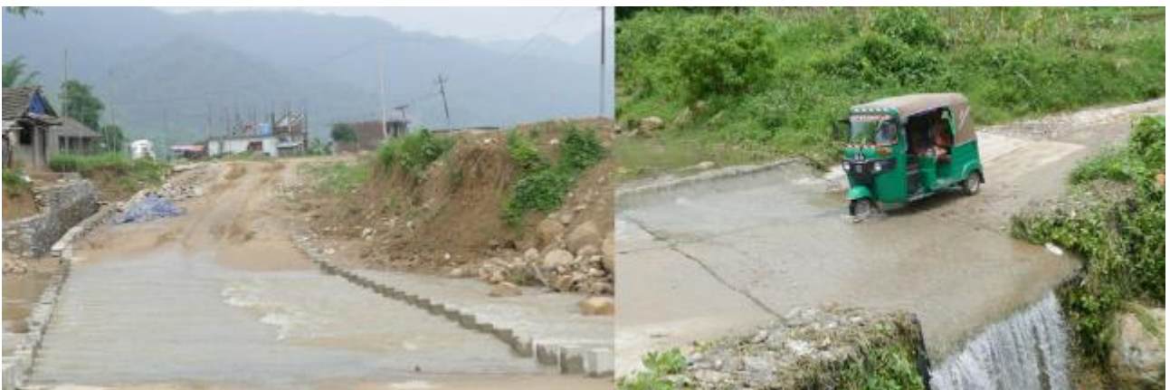
Figure 28 Concrete drifts on the road
