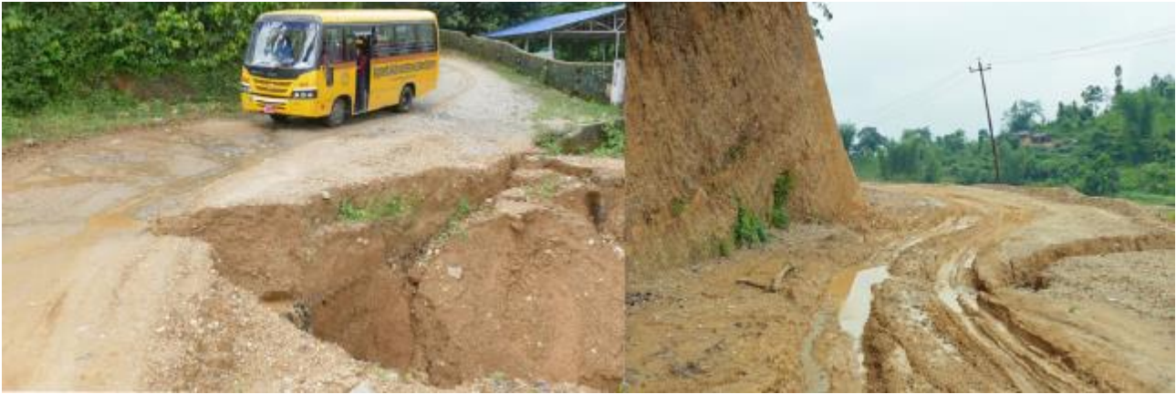
Figure 31 Gully erosion threatening parts of the road
