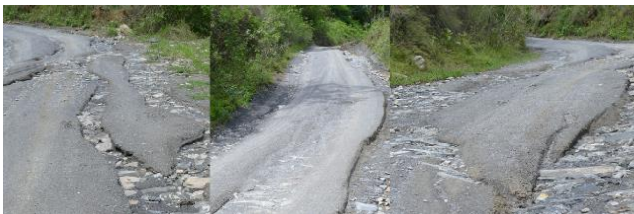
Figure 16 Recently laid but eroding stone-waste surface placed on top of stone soling near the quarry
