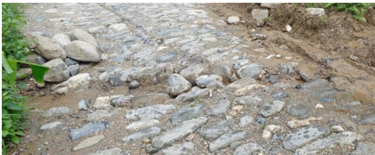
Figure 33 Cross-drain created by farmers wanting irrigation water on other side of the road
