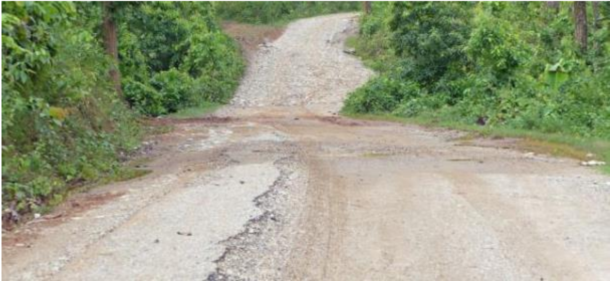
Figure 21 Part of section 1 showing some remaining Otta seal (foreground) and a cobbled slope (behind)
