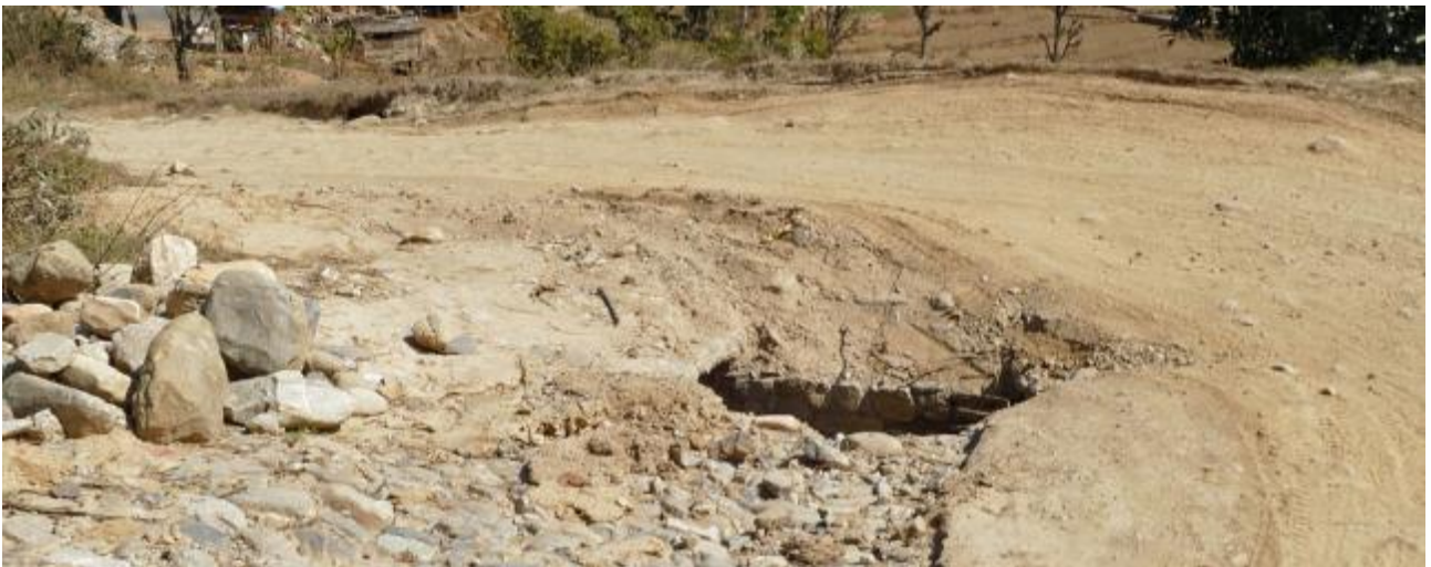
Figure 27 Failed cross-drain culvert on cobblestone bend
