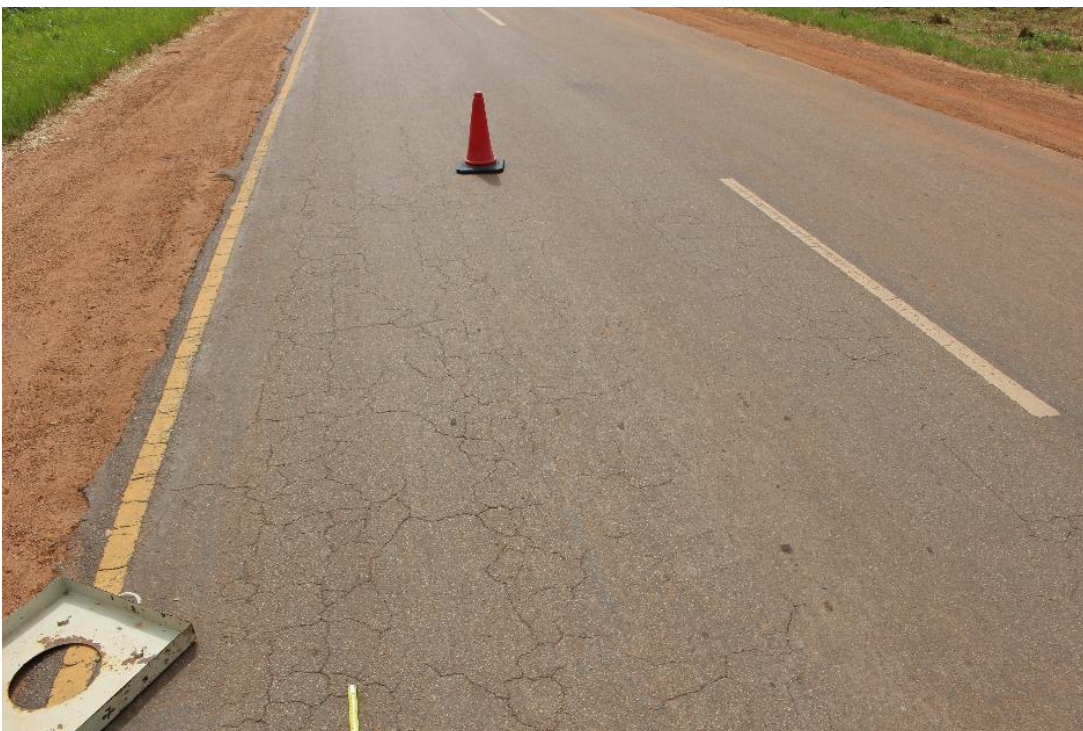
Figure 6 Wheel path cracking on Samfya – Musaila (Section 1)
