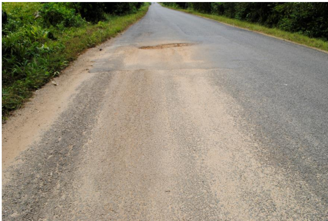
Figure 9 Rutting and cracking on Mpataba Junction – Half Asini (Section 1)
