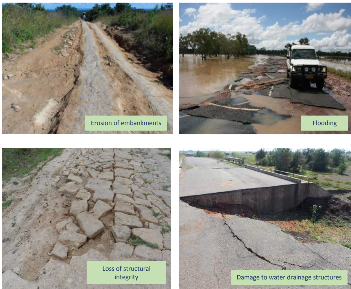
Figure 5 Damage to road infrastructure due to climate-related environmental stresses
