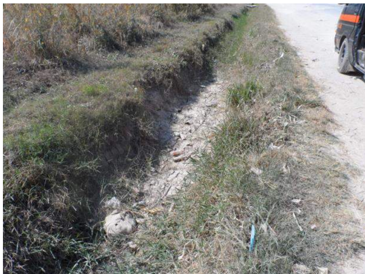
Figure 12 Evidence of ponding of water in side drain
