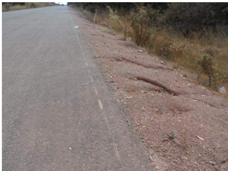
Figure 27 Poor finish of newly constructed road
