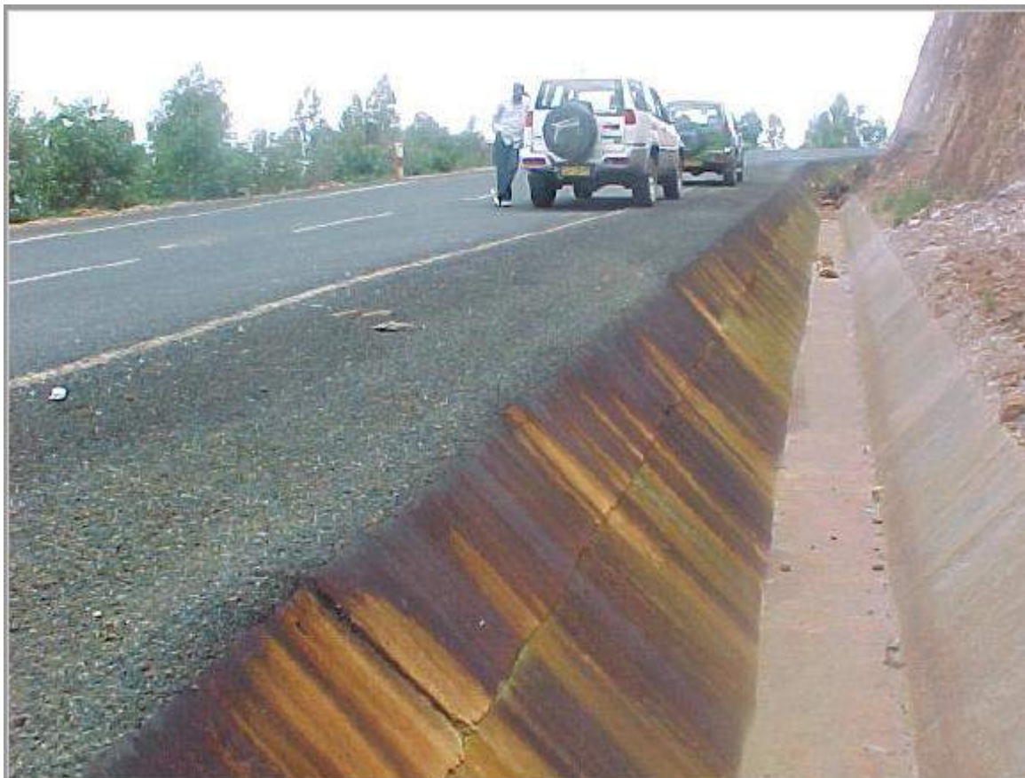
Figure 9: An example of yellow/brown staining of a concrete side drain due to the presence of sulphides
