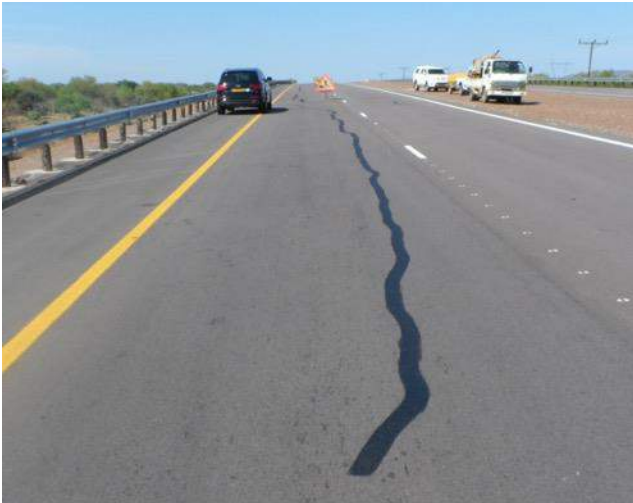
Figure 25 Cracking of embankment due to overstressing
