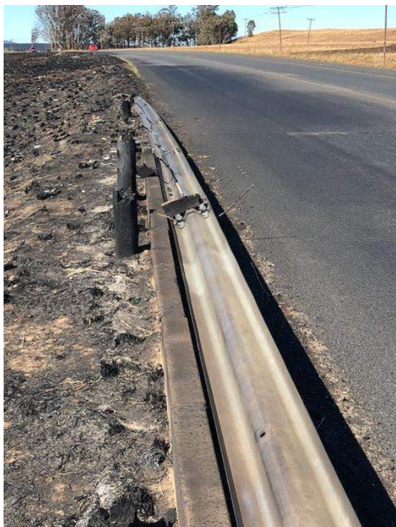
Figure 31 Damage to guardrail posts and bitumen surfacing caused by wildfire
