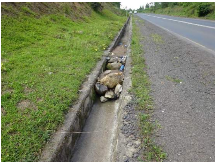
Figure 16 Unpaved area between impervious seal and lined drain allowing access of water into the pavement (Note poor maintenance of side drain as well)
