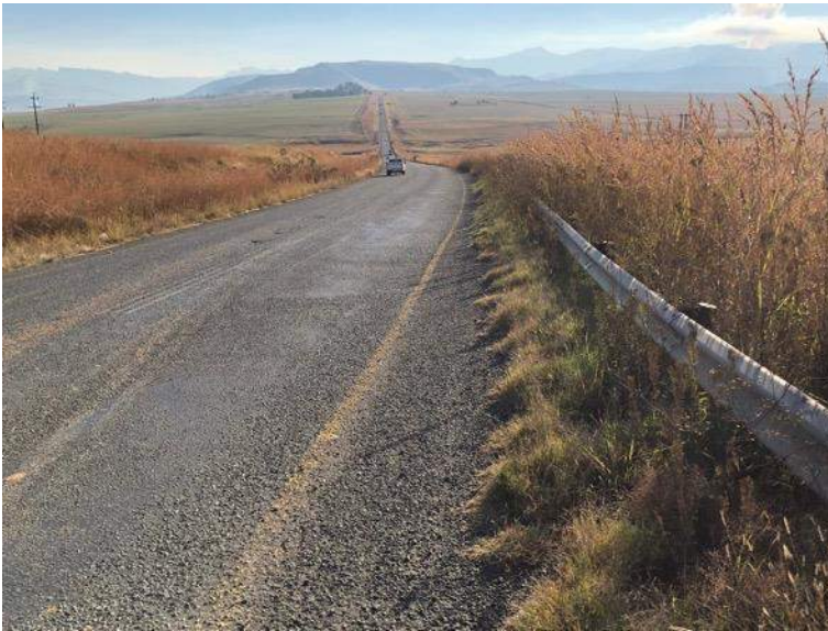
Figure 29 Thick vegetation alongside road indicating insufficient maintenance (rated at 5/5)
