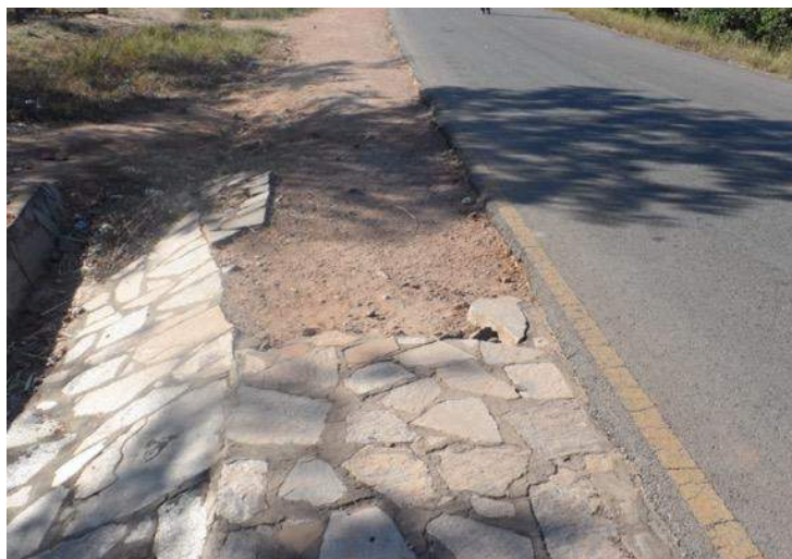
Figure 28 Poor finish of protection works resulting in failure – no “anchor” beams
