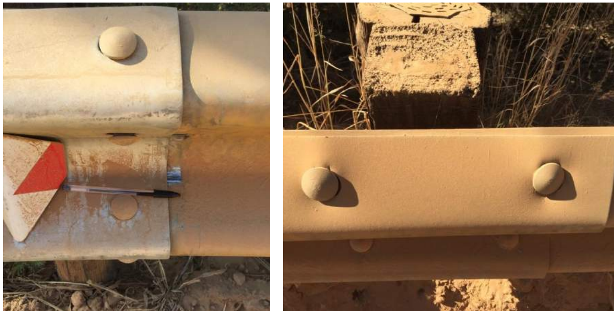
Figure 41 Effect of expansion of metal guard rails: a) loosely tightened and b) tightened so as to avoid thermal movements and cause deformation (daily movement visible in left photograph)
