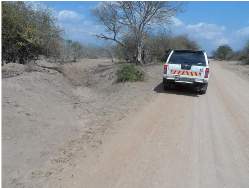
Figure 34 Short mitre drain that is unable to dissipate collected water effectively
