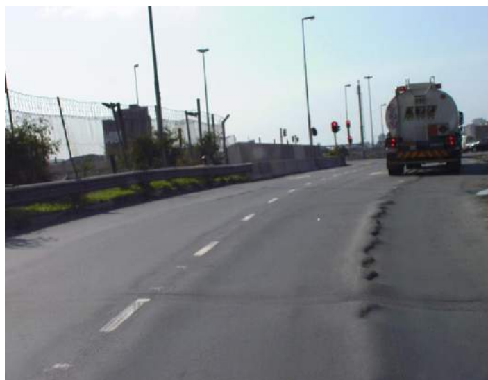
Figure 11 Rutting and deformation of asphalt resulting from high temperatures and traffic loading
