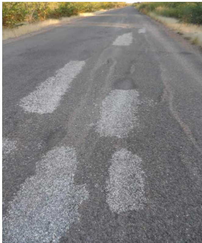
Figure 29 Example of recurring distress in embankment due to highly dispersive soil used as the fill material
