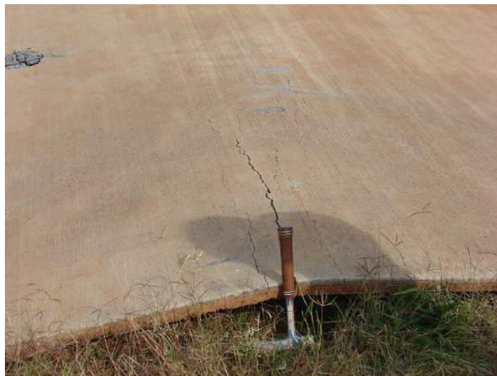
Figure 13 Lifting of thin continuously reinforced concrete road resulting from thermal expansion
