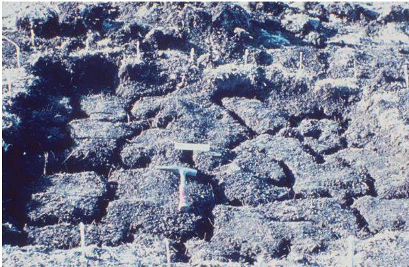
Figure B.1 Typical evidence of the presence of expansive clay soils
