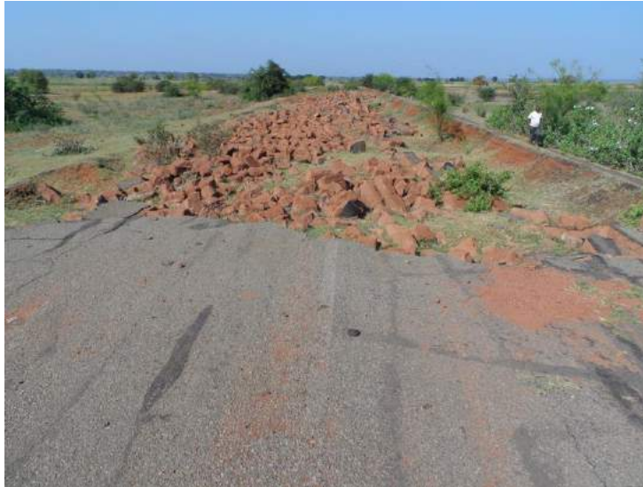
Figure 19 Complete loss of embankment and road due to turbulent flow conditions during overtopping and weak subbase
