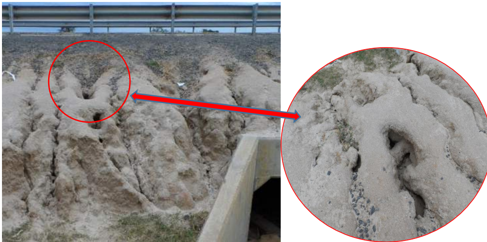
Figure B.3 Dispersive soil showing formation of “pipes”
