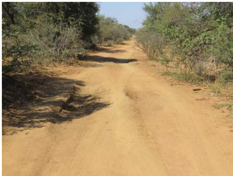
Figure 5 Typical un-engineered earth road showing damage caused by water retention
