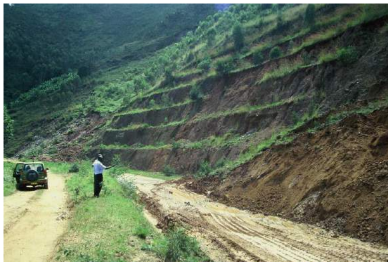
Figure 15 Road closure due to slope failure. Note deviation on the left created to by-pass the failure
