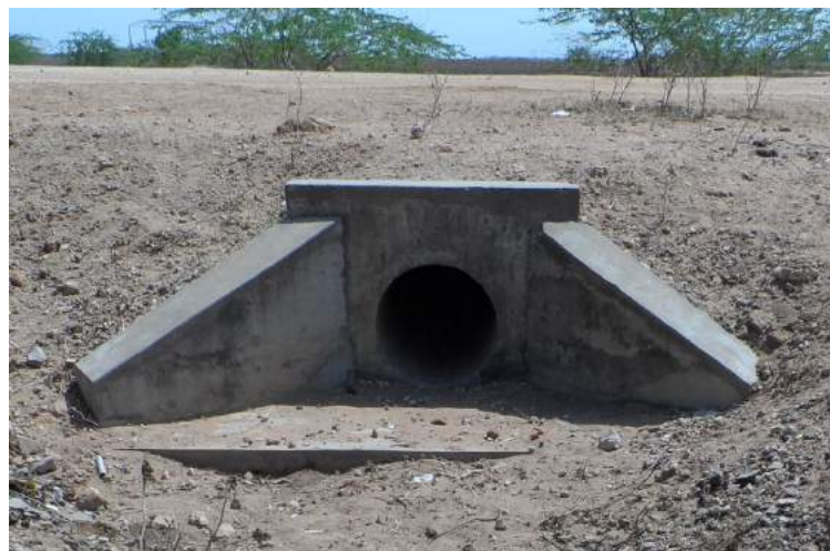
Figure 39 Separation of wing-walls from headwall on relatively new culvert
