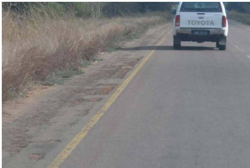
Figure 10 Deterioration of single chip seal shoulder compared with double chip seal on carriageway
