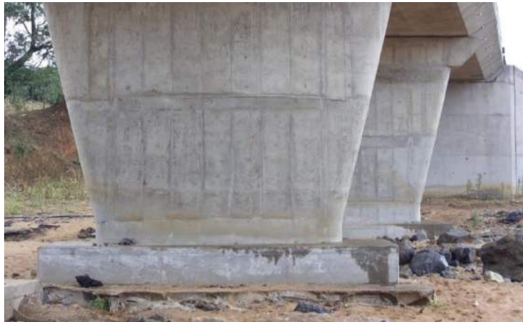
Figure 38 Localised scour around bridge pier footing
