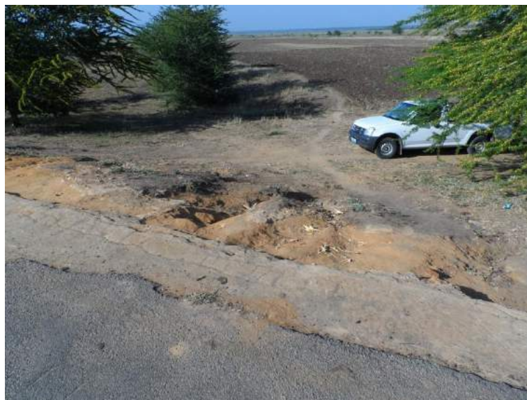
Figure 23 Erosion caused by access of vehicles, pedestrians and animals off the road
