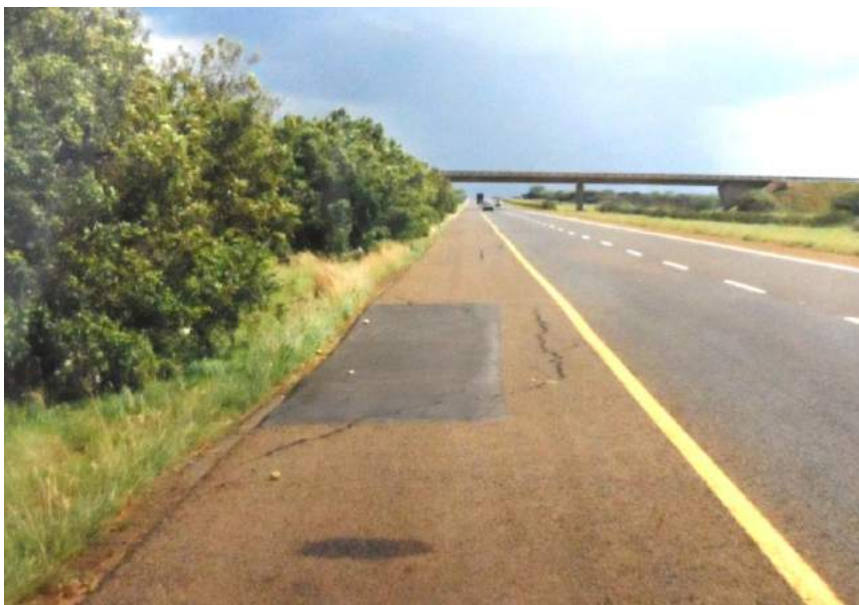
Figure 28 Example of cracking due to dehydration caused by trees next to road leading to subsidence in excess of 150 mm in patched area
