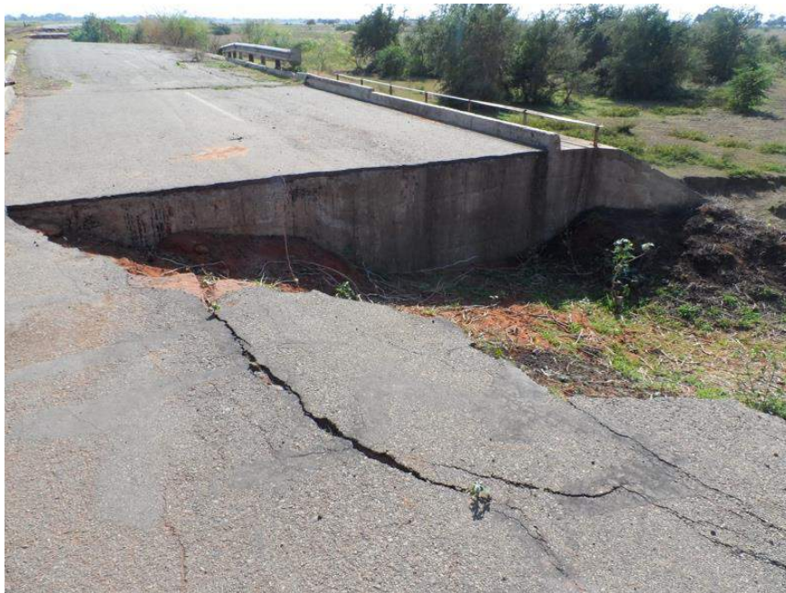
Figure 35 Flood damage to bridge abutment after overtopping of embankment
