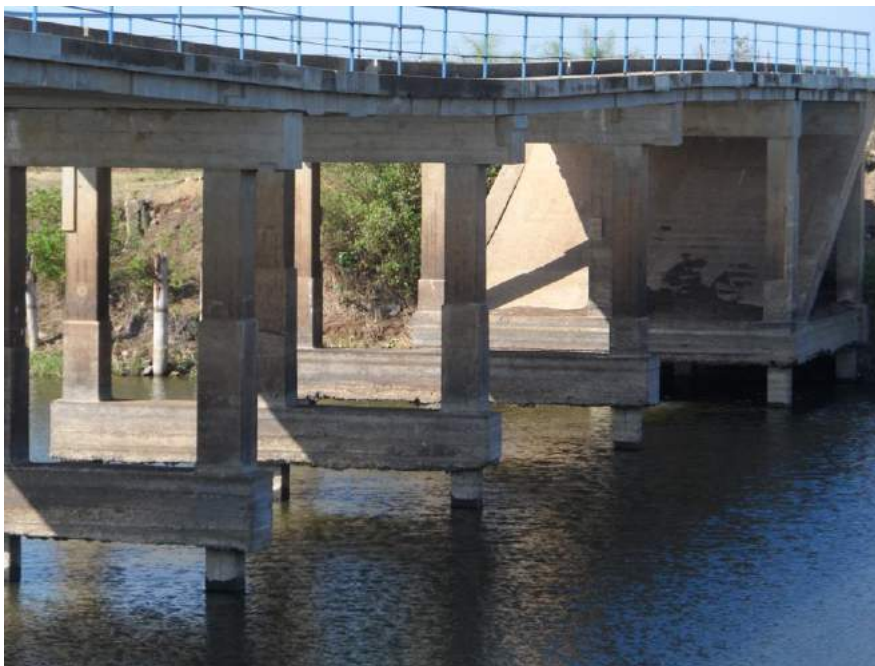
Figure 37 Subsidence of bridge deck due to scour damage of support pier
