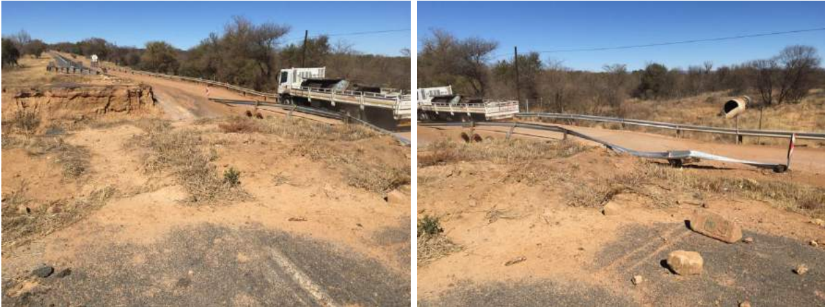
Figure 36 Damage to steel culvert after storm with total loss of embankment. Photograph on right shows final location of metal pipe
