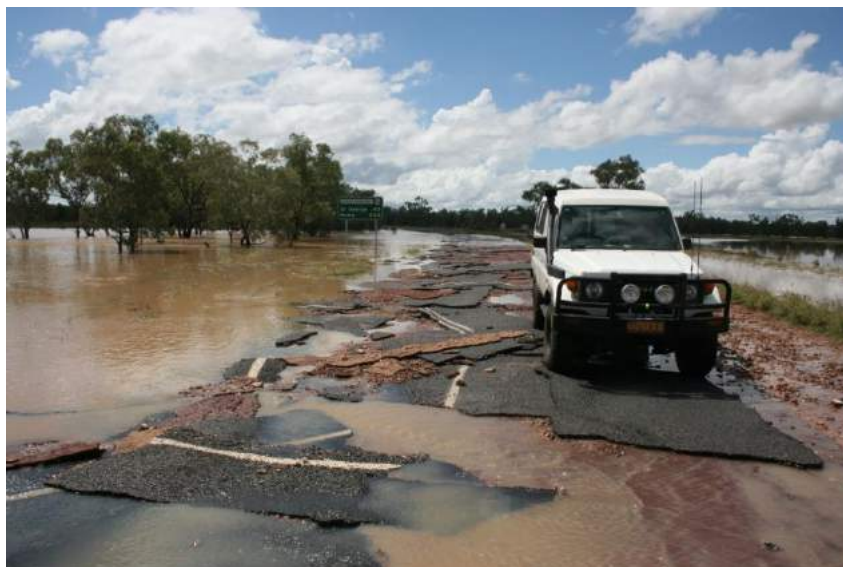
Figure 9 Loss of surfacing caused by high uplift pressures during flooding 12
