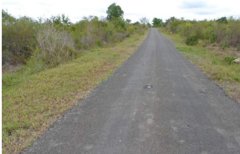
Figure 30 Grassed and built-up shoulders negating effectiveness of drainage from road surface
