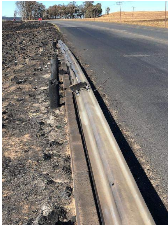
Figure 40 Damage to guardrail posts and bitumen surfacing caused by wildfire
