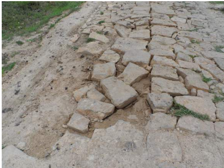
Figure 14 Damage to hand-packed stone road after flooding
