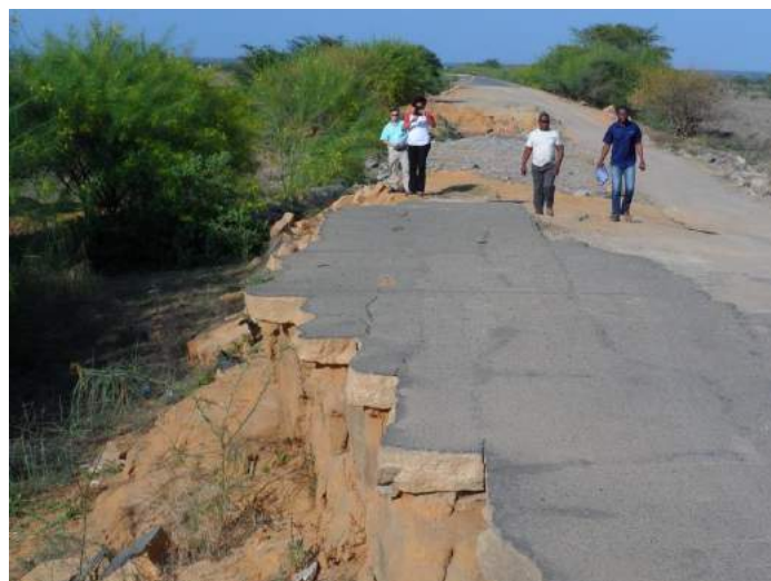
Figure 18 Undercutting and collapse of pavement due to erosion of embankment
