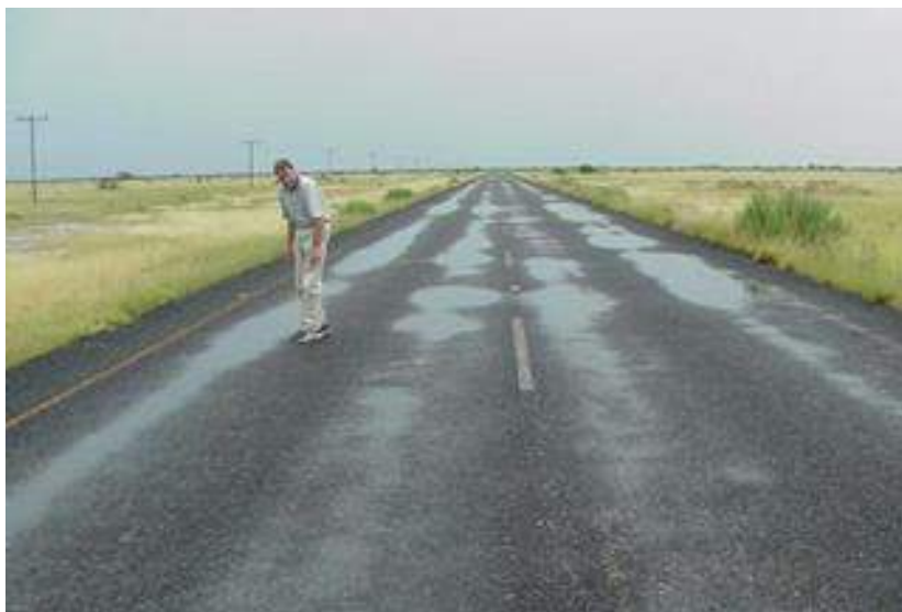
Figure B.6 Typical manifestation of collapsible subgrade
