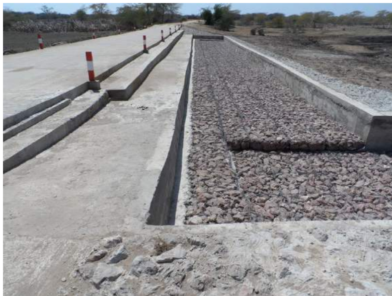
Figure 22 Complex concrete ford with water velocity controllers and stilling pond
