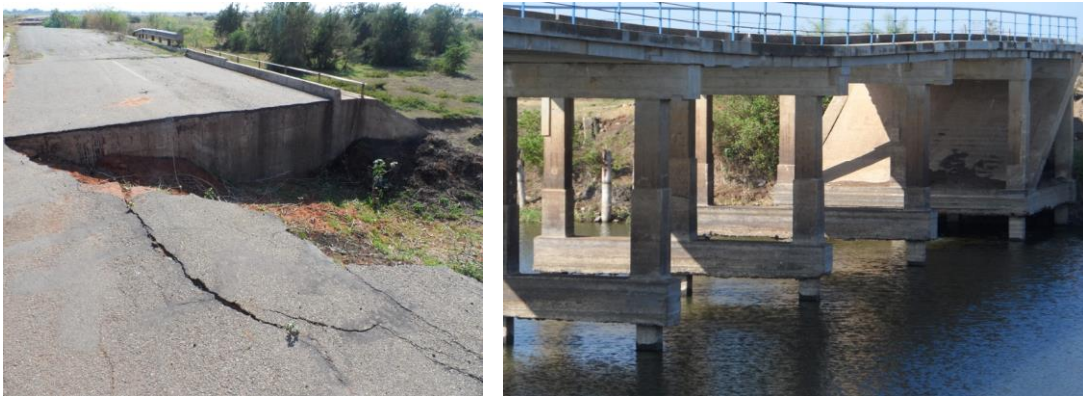
Figure 8 Flood damage on approach to bridge and to bridge structure
