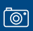
Trial placement of the first modular bridge component, manufactured off site and brought to the Interchange site in Solihull by road, 2020.
