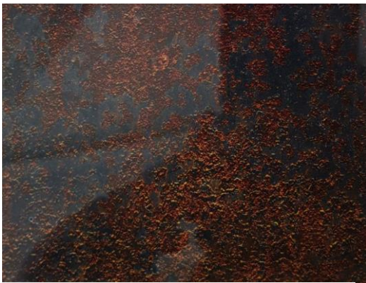
Figure 1.3 Rust Grade A
