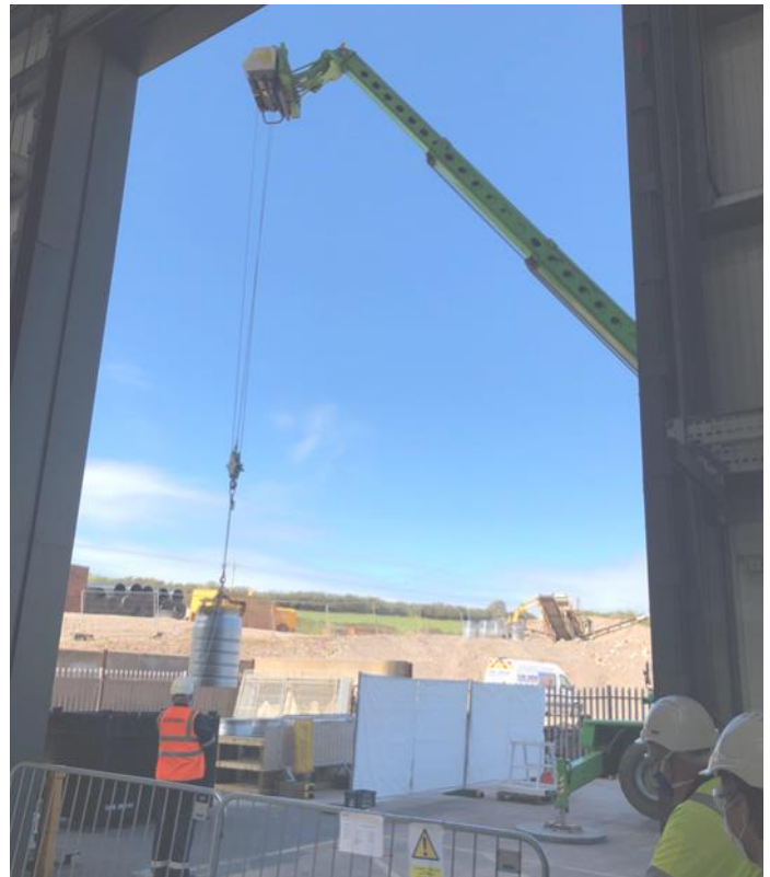
Practice makes perfect: off-site trials run through the disposal of drums. Above: a mock-up of drum removal from train at LLWR site, and below, emplaced in 'Vault 8'
