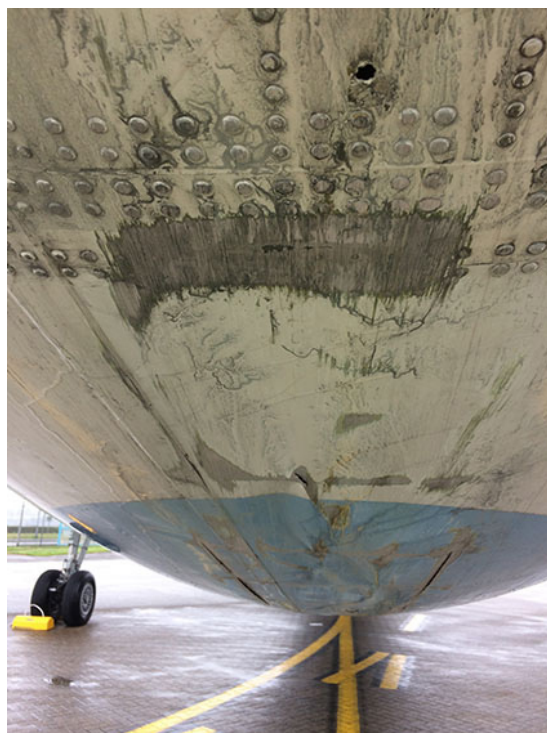
Figure 2 Damage to aft fuselage
