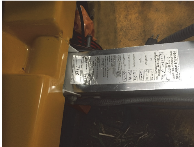
Figure 2 Damage to base tube
