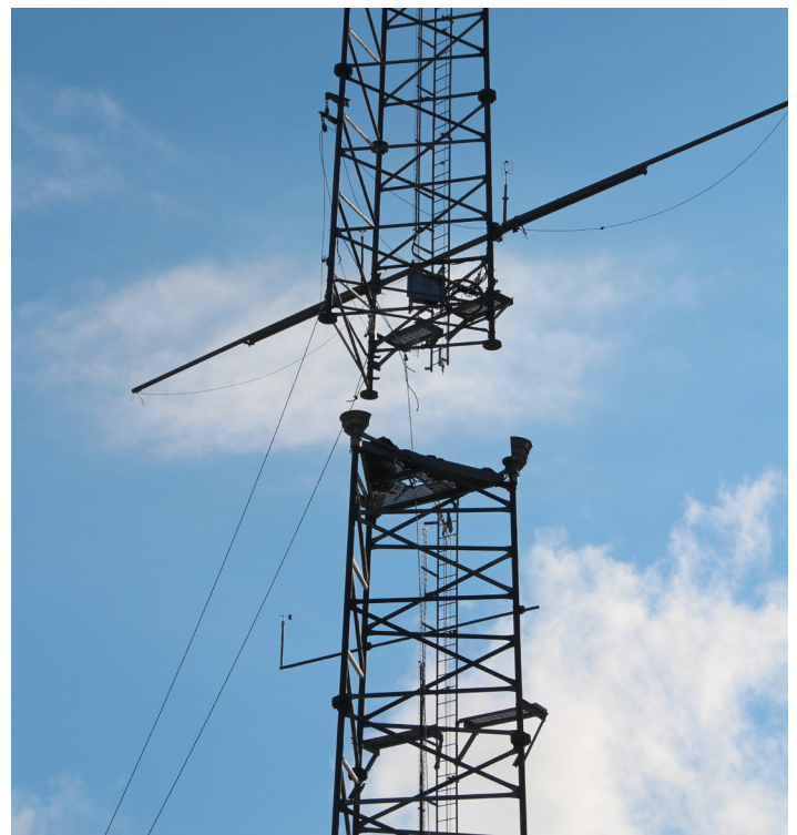
Landing the upper tower section with the use of guide cones and video cameras.
