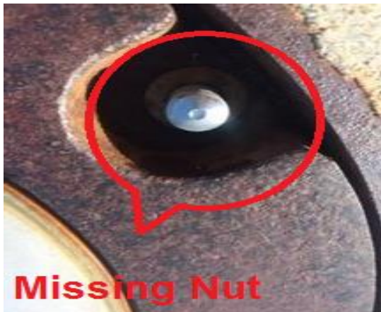
Photograph – 01: Missing Nut
