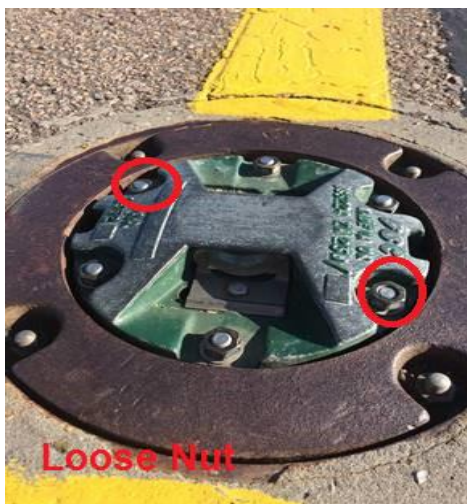
Photograph – 03 : Loose Nuts
