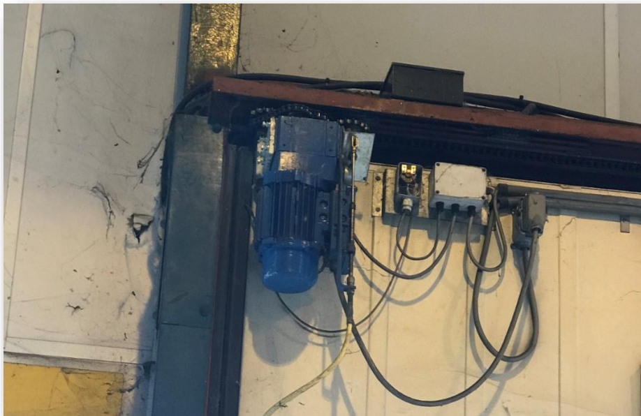
Photo 3 Showing Motor Suspended under Door Frame
