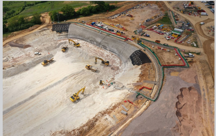
Image of the excavation of the south portal tunnelling machine launch site (due to be launched early next year), HS2 Ltd
