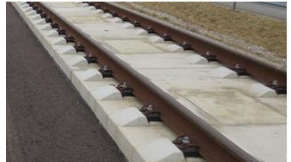
Non-ballasted slab track
