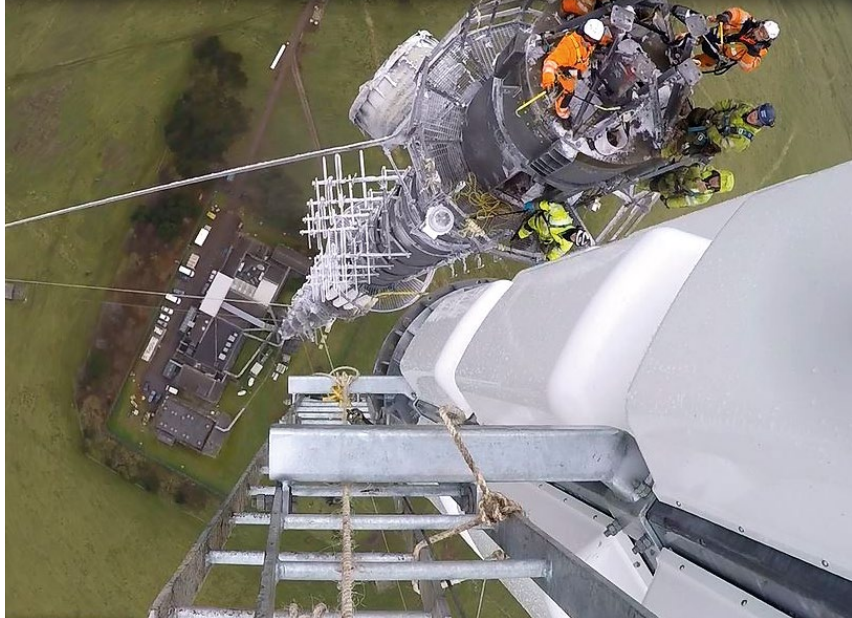
Helicopter lifting new 700MHz antenna into position at top of Mendip TV mast in Somerset; DCMS.
