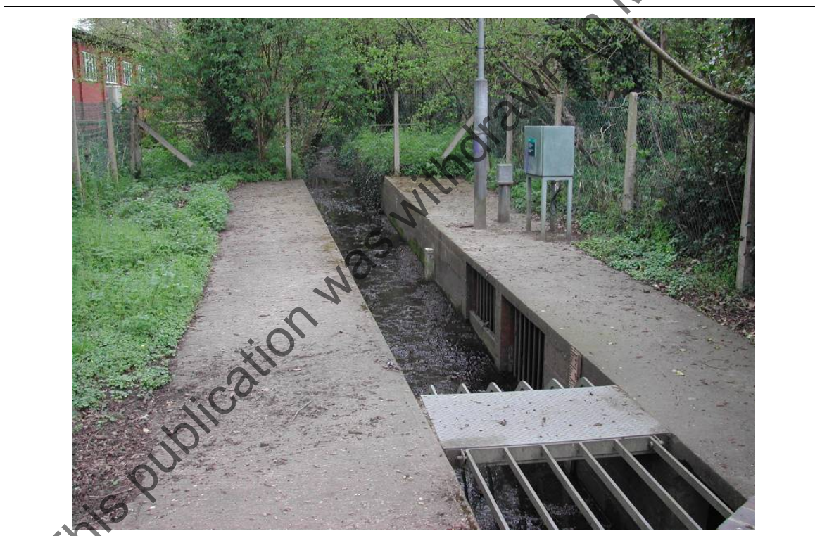
Figure 12.1 Kydbrook screen and bypass facility, Ravensbourne, South London.
