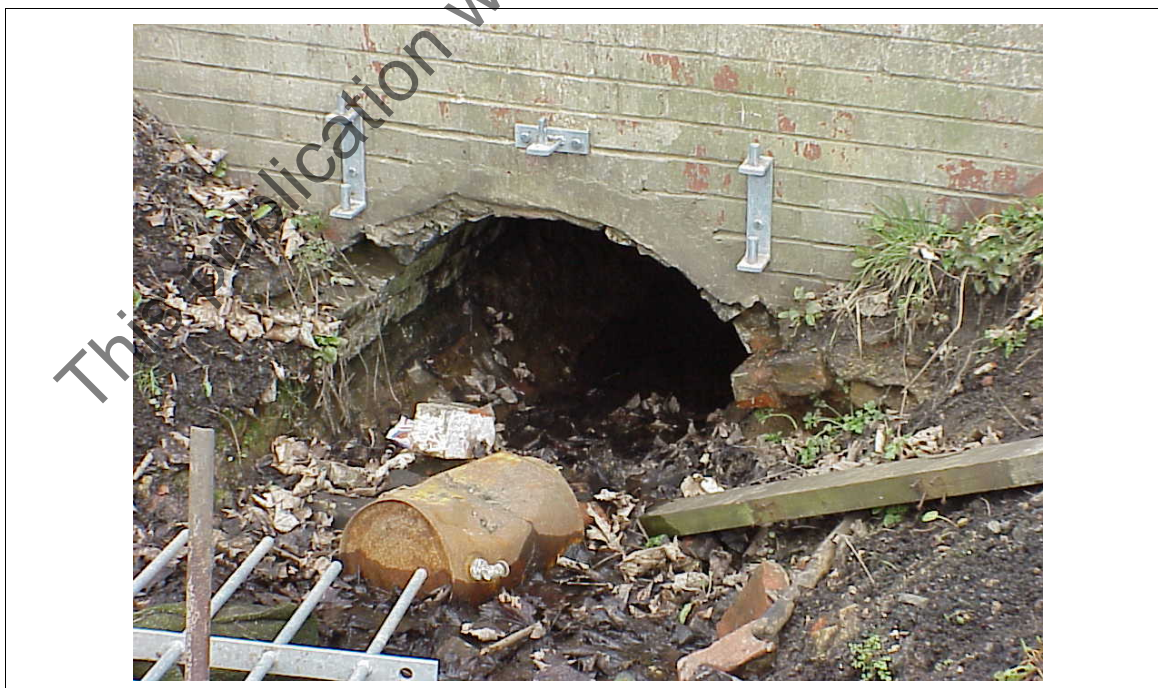
Figure 4.3 Screen on a small culvert not securely fixed in place.
