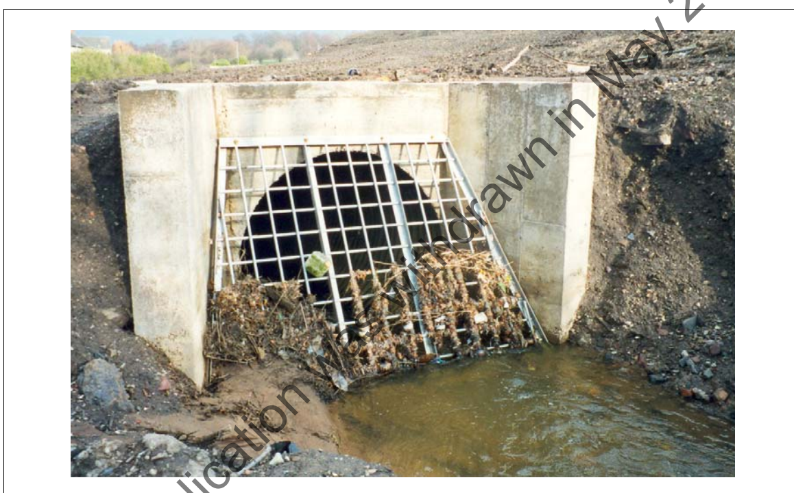
Figure 4.2 Poorly designed screen.
