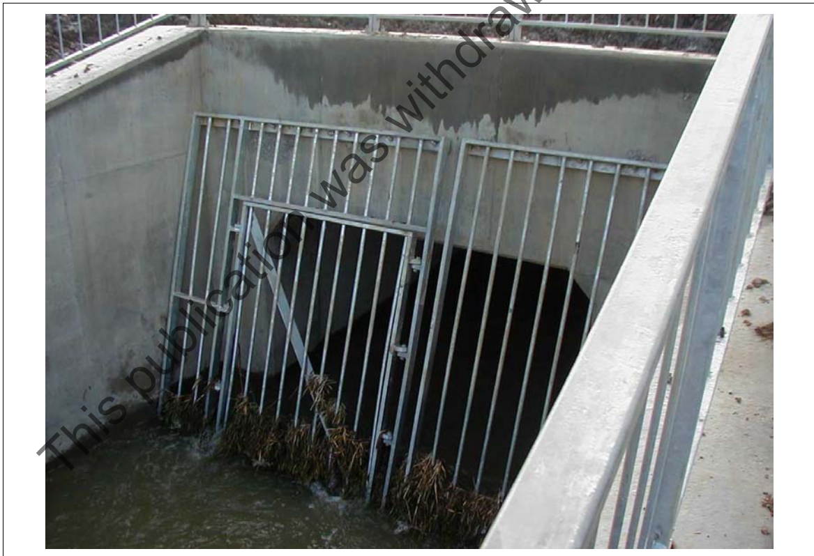
Figure 4.5 A security screen on the outlet of a culvert.
