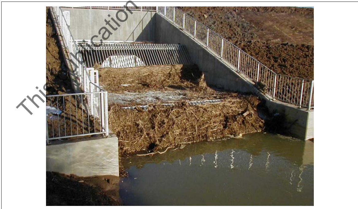
Figure 7.5 Multi-stage screen at the outlet from a flood storage facility.
