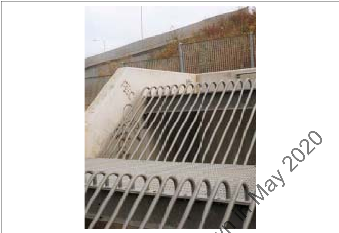
Figure 8.2 Design tolerances allowed children to squeeze between the concrete sidewall and the end bar on the screen.
