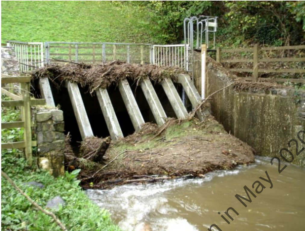
Figure 8.1 Coarse screen at a flood relief culvert inlet showing degree of debris build-up (the 'Beaverscreen' effect).
