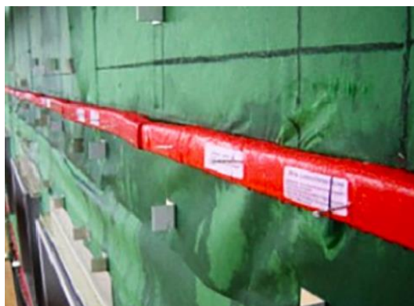
Figure A4 – Intumescent cavity barrier during installation in a ventilated cladding system [1]
