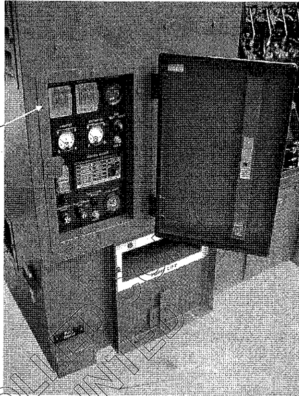
Fig 3 Control panel and door
