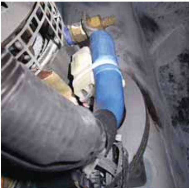
Figure 1 – Bow thruster showing exposed power cables and fire damage
