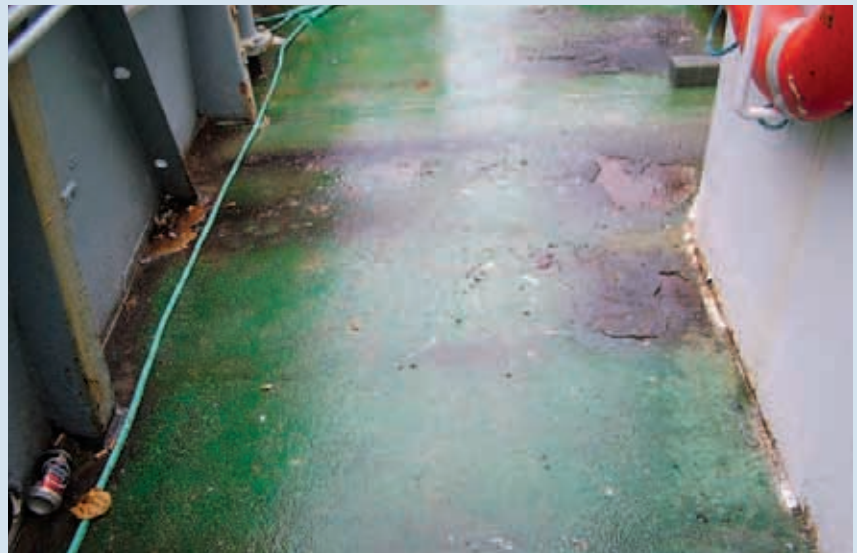
Figure 2: Blistering of the paint on the main deck
