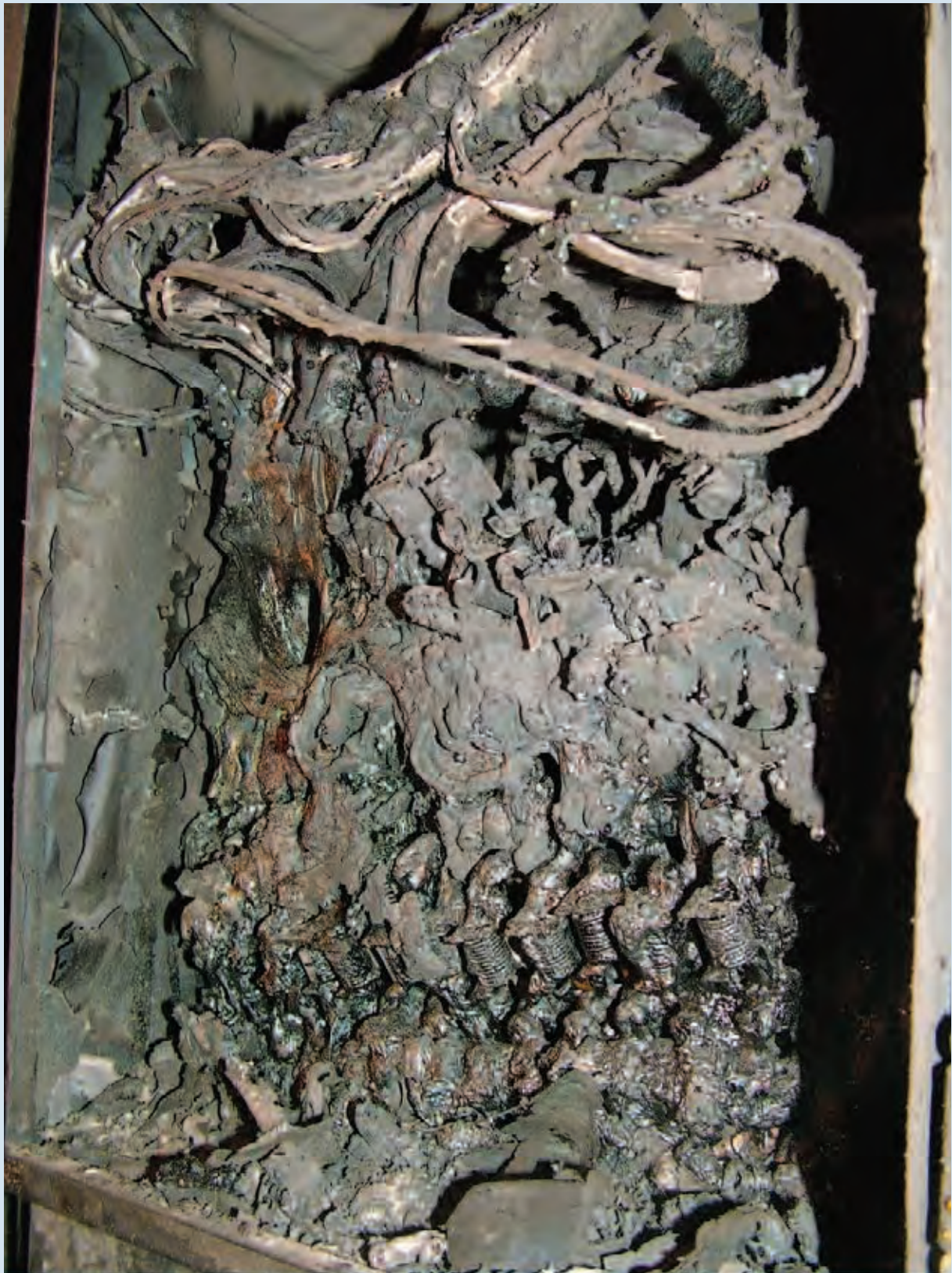
Figure 5: Damage to the 220v distribution panel
