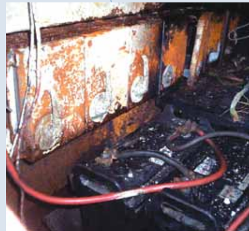
Damaged area above batteries.
