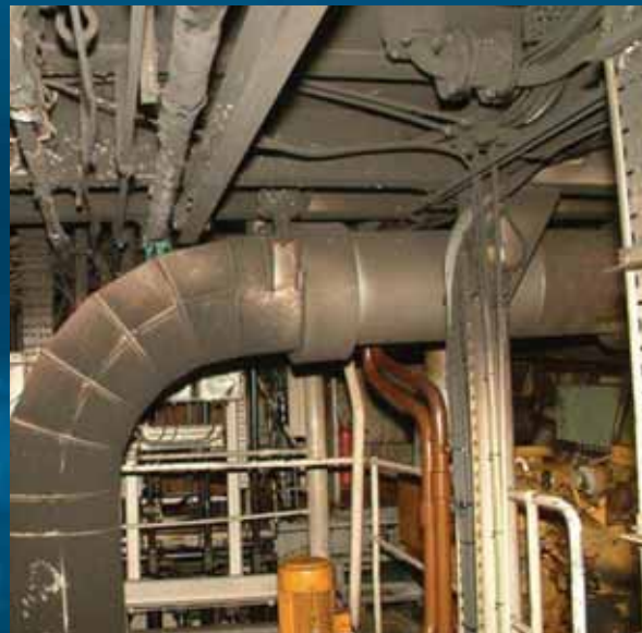
General smoke damage.
