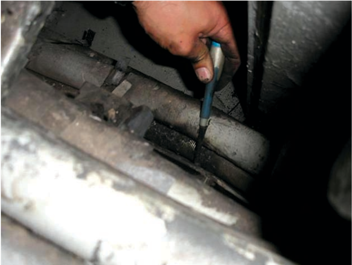
Figure 2: Charred rubberised sheathing of cable
