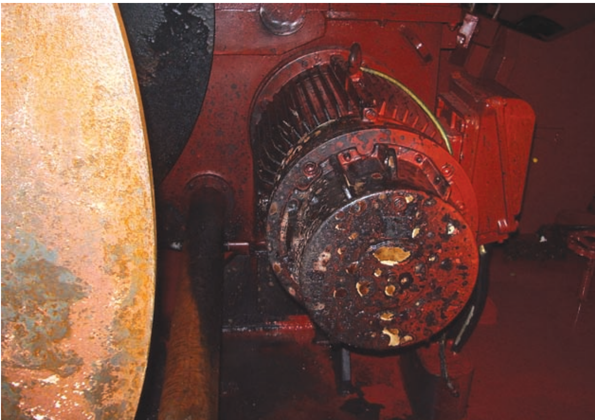
Figure 5: Winch motor damage
