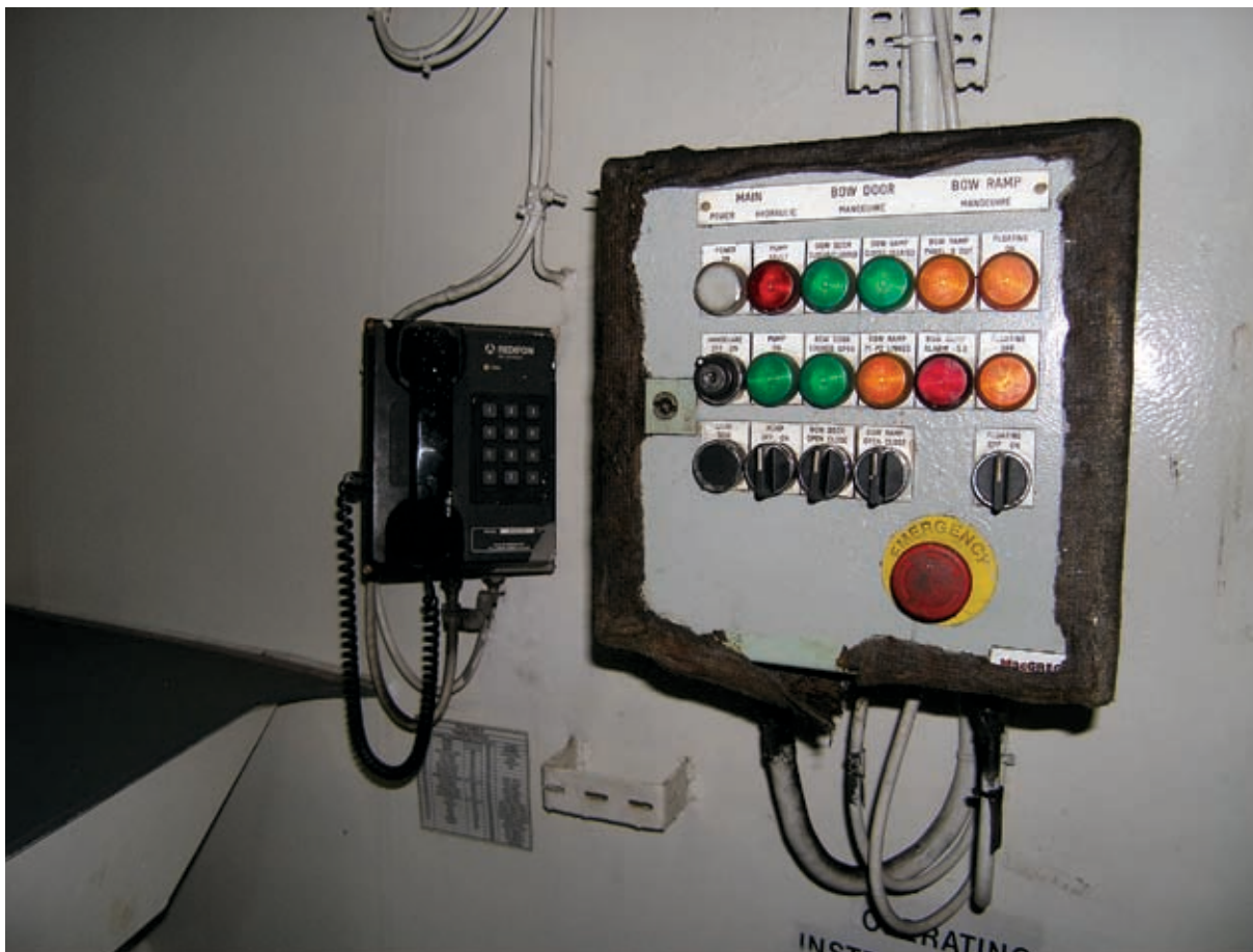
Figure 2: Bow door operating panel on car deck
