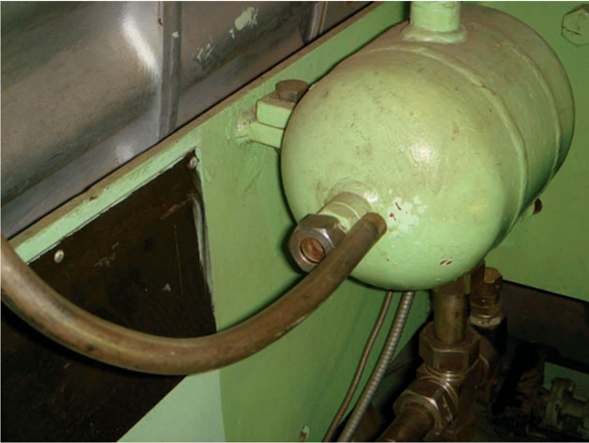
Figure 3: Pipe disconnected from reservoir connection fitting
