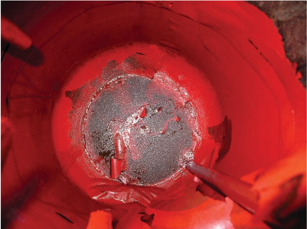
Damage inside the water tank
