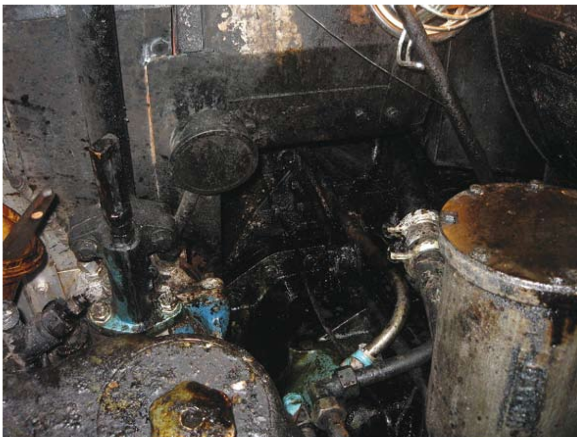
Figure 1 – Burst fuel pipe
