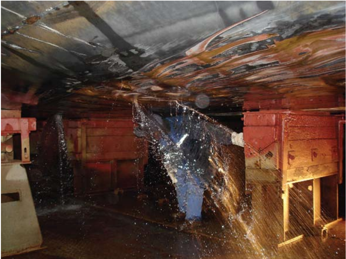
Damage below the waterline
