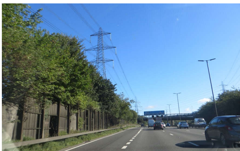
Figure 5-3 Example of environmental barrier in poor state of repair (SB approaching J7)
