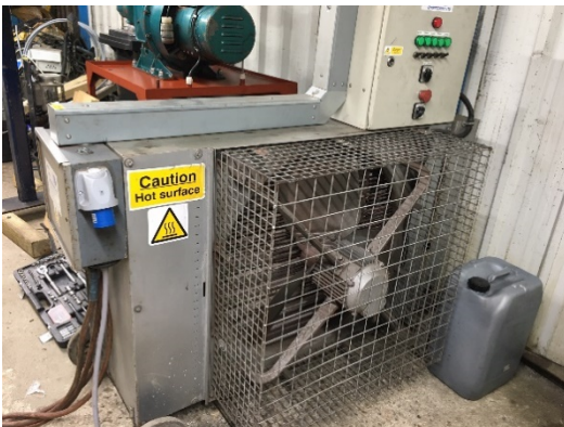
Figure 27 - Spare load bank
