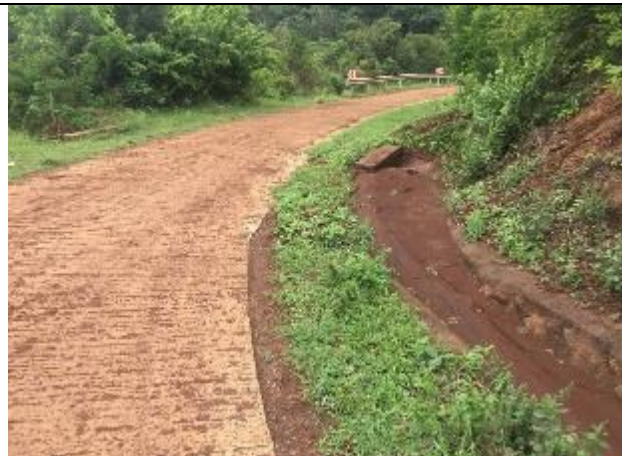
Good performing lightly reinforced concrete (75 mm) section, but severe sedimentation build-up
