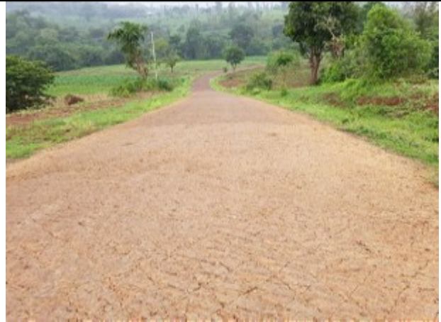
Good performing Geo-cell section, poor maintenance in side drains
