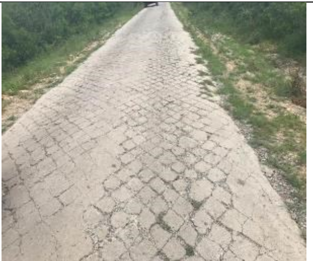
Geocell sections : Severe rutting in one wheel path
