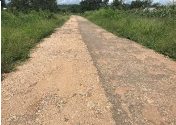
Sand seal section: Lime slurry seal (LHS) vs. Cement slurry seal (RHS)
