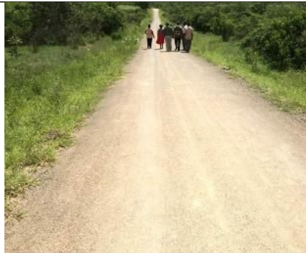
Good performing double seal section, but drains are covered by shrubs, tall grass – lack of maintenance
