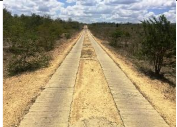
Good performing concrete, but severely eroded gravel shoulders
