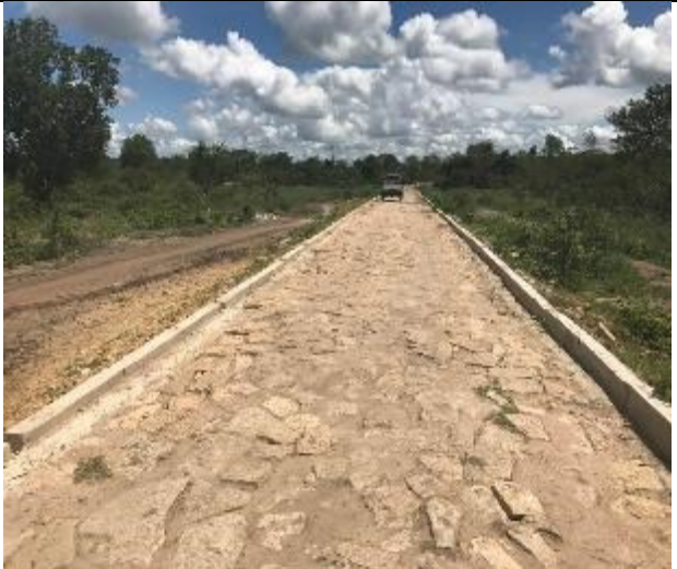
Hand-packed stone section: Surface deformations and loss of stones
