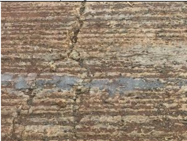
Unreinforced concrete slab (100 mm) section: Severe longitudinal cracks
