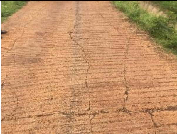
Unreinforced concrete slab (75mm) section: Dominance of both longitudinal and transverse cracks (block cracking)
