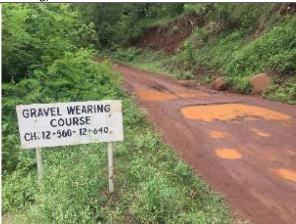
Gravel wearing course section: Large potholes and associated water ponding
