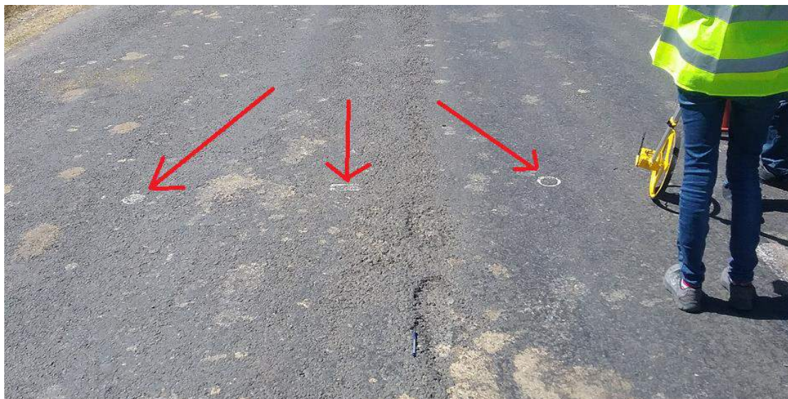
Figure 2-3: Worn out Marks of the LTPP sections
