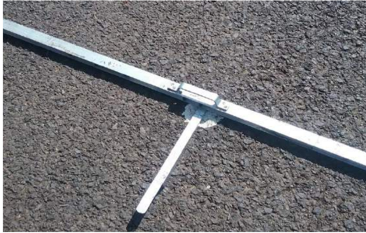
Figure 4-2: Rut depth measurement using 2m standard straight edge and measuring wedge.
