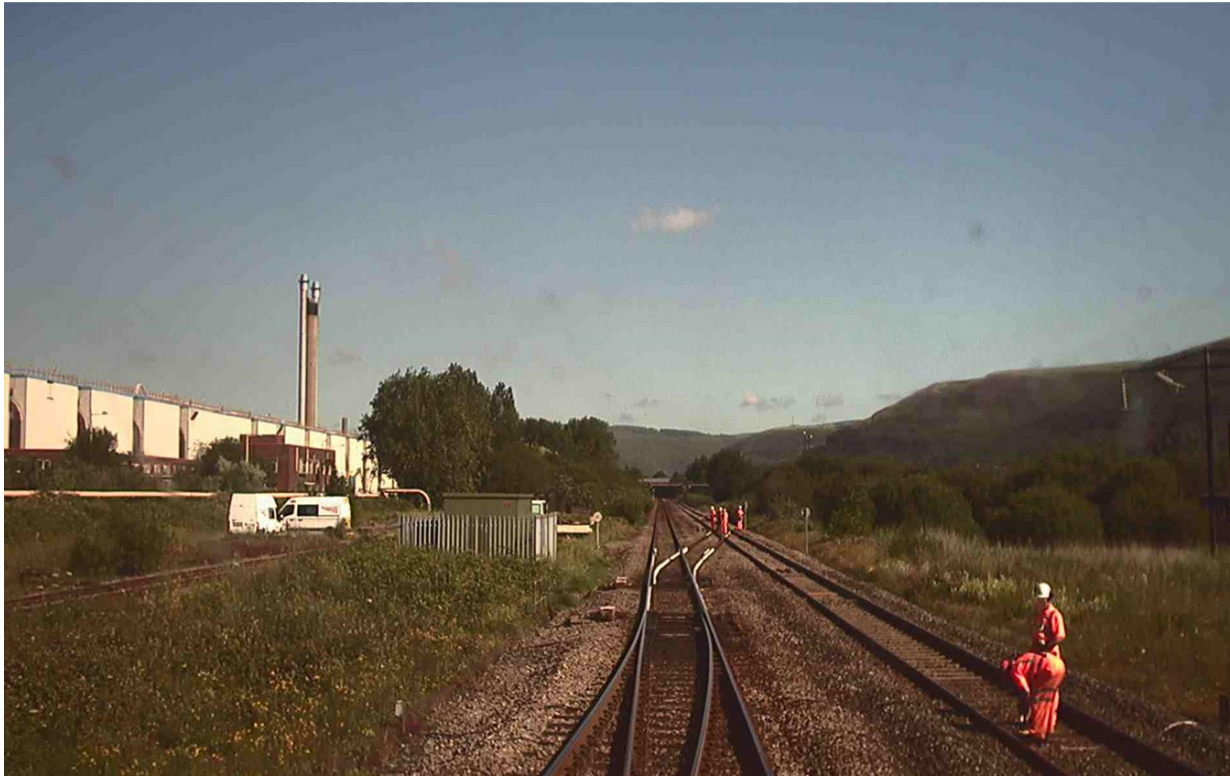
Figure 3: FFCCTV image looking towards Port Talbot from a train on the down main line at approximately 09:24 hrs, showing the two groups working on the open up main line approximately 100 metres apart
