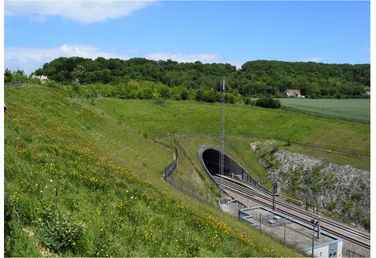
Numerous fencing runs around portal; some requested by Structures Examiners following their annual inspection
