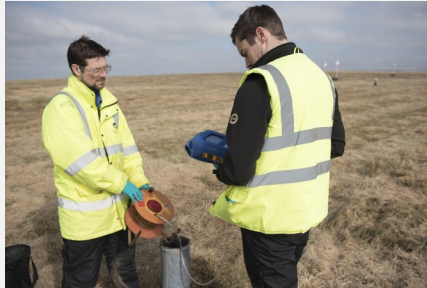
Teamwork: James Ridehalgh, left, and colleague Andy Scott, monitoring on the trench cap
