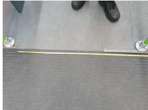
Figure 9: Top down view of floor obstruction.
