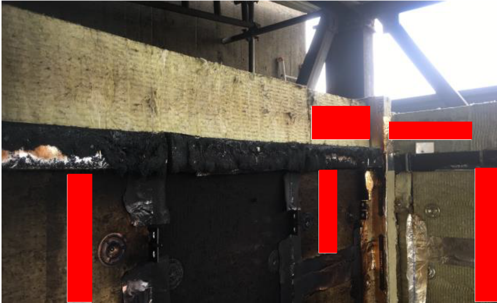
Figure 13 – 4 th cavity barrier (top) from main wall following removal of the rainscreen
