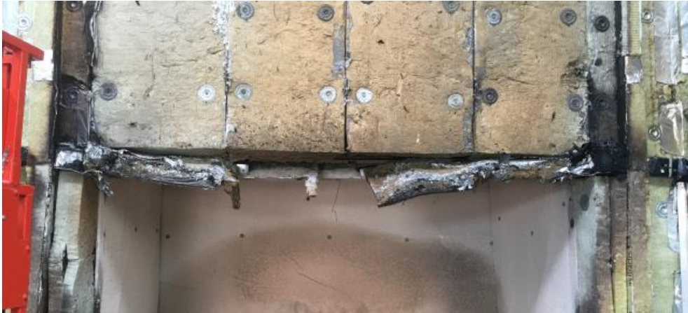
Figure 7 – 1 st cavity barrier (directly above burn chamber) from main wall following removal of the rainscreen
