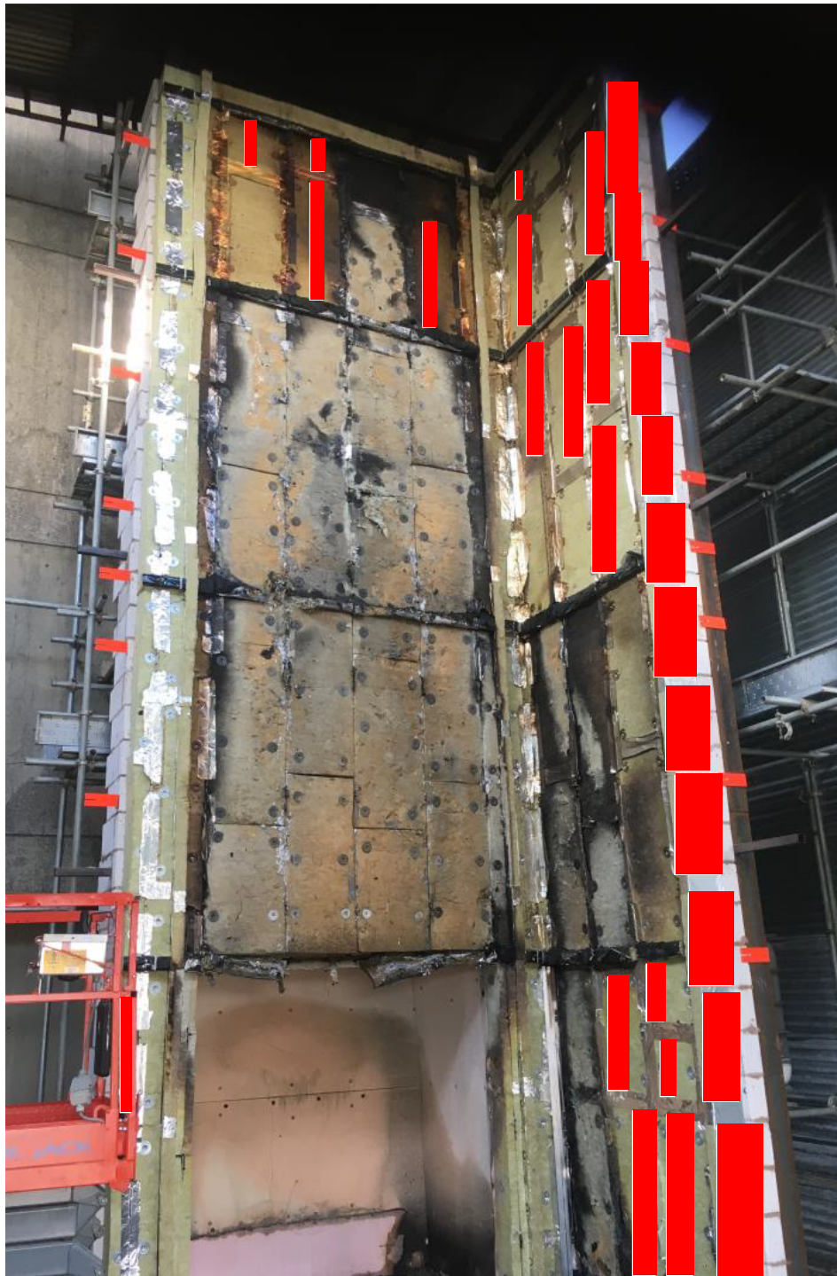
Figure 6 – Insulation board and cavity barriers following removal of the rainscreen and support rails
