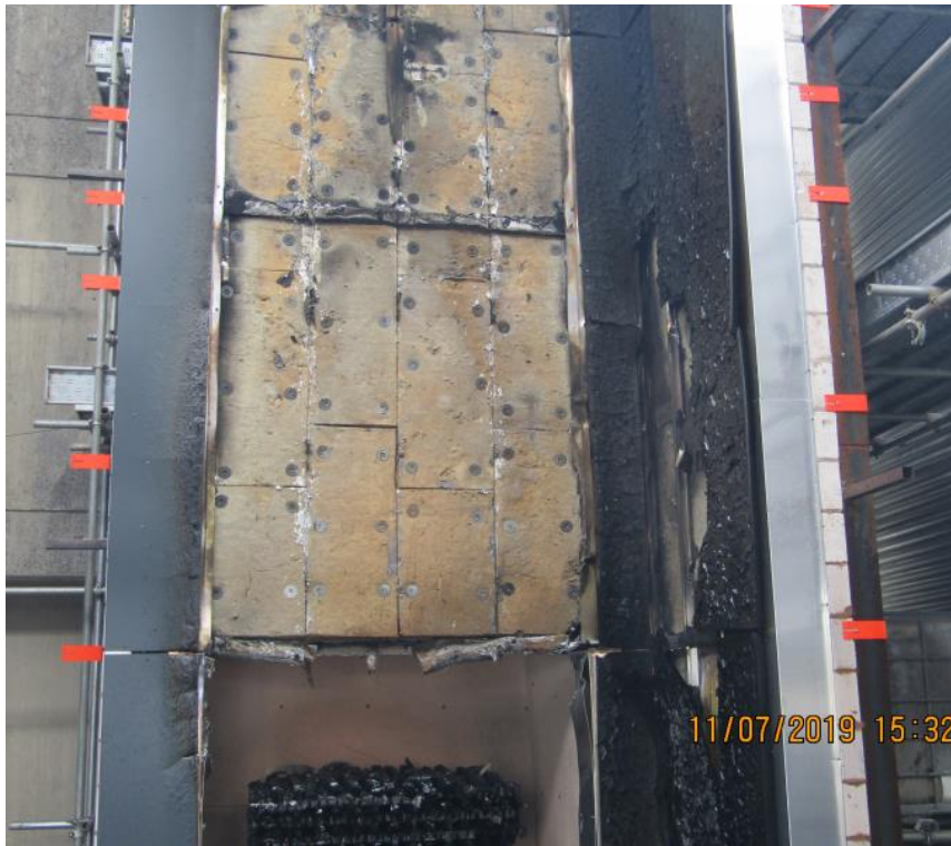
Figure 4 – Area directly above combustion chamber post test
