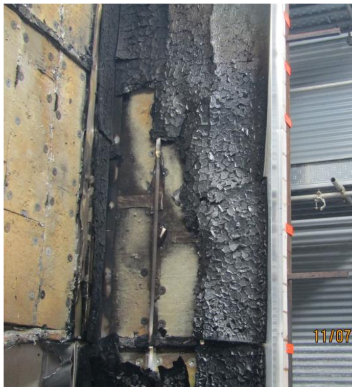
Figure 5 – Return wall above combustion chamber post test
