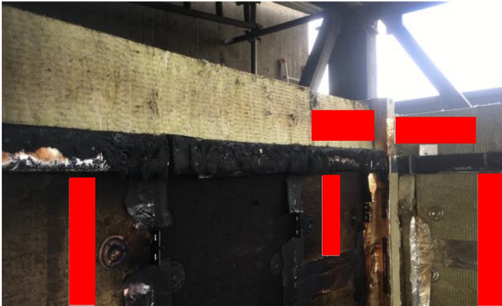
Figure 30 – 4 th cavity barrier (top) from main wall following removal of the rainscreen
