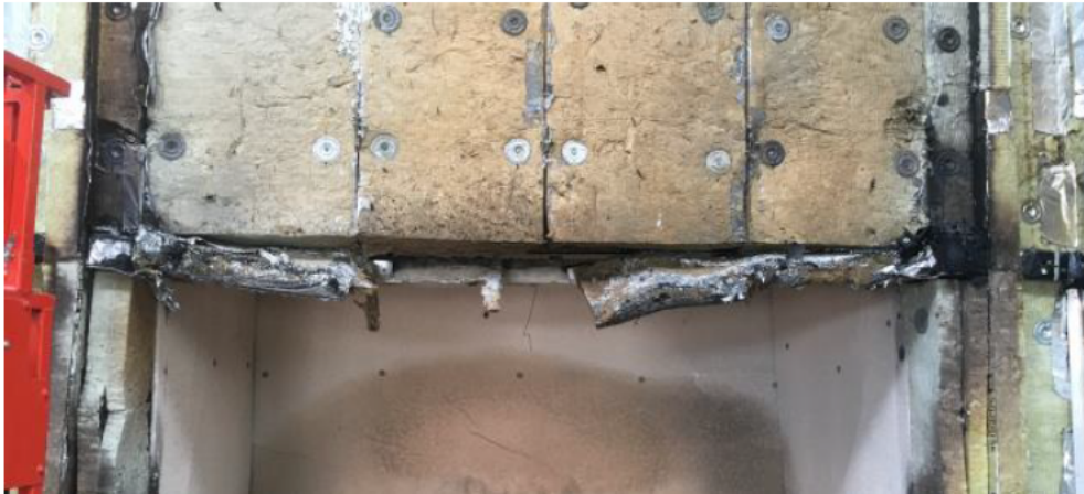
Figure 24 – 1 st cavity barrier (directly above combustion chamber) from main wall following removal of the rainscreen
