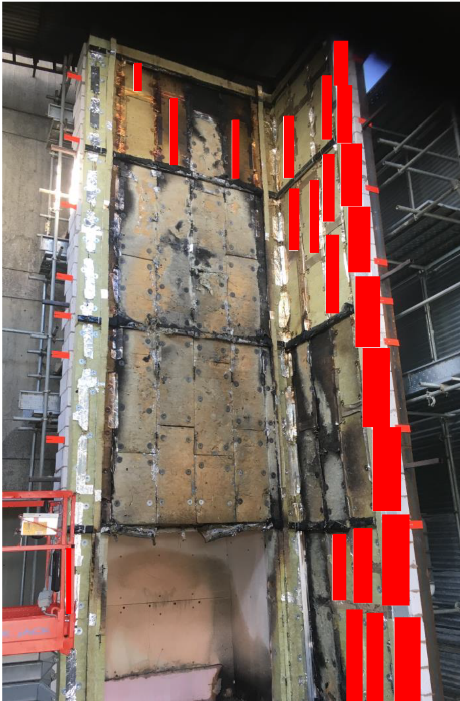
Figure 23 – Insulation and cavity barriers following removal of the rainscreen and support rails
