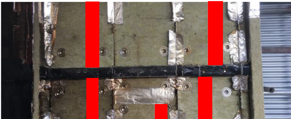
Figure 29 – 3 rd cavity barrier from return wall following removal of the rainscreen
