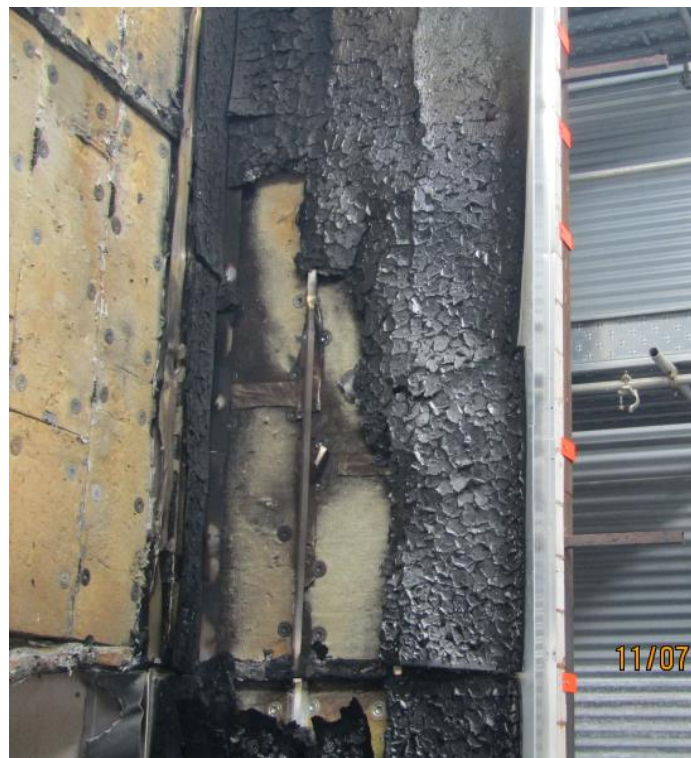
Figure 22 – Return wall above combustion chamber post test
