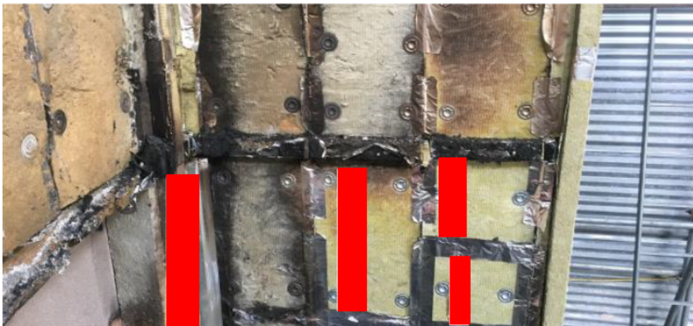
Figure 25 – 1 st cavity barrier (directly above combustion chamber) from return wall following removal of the rainscreen
