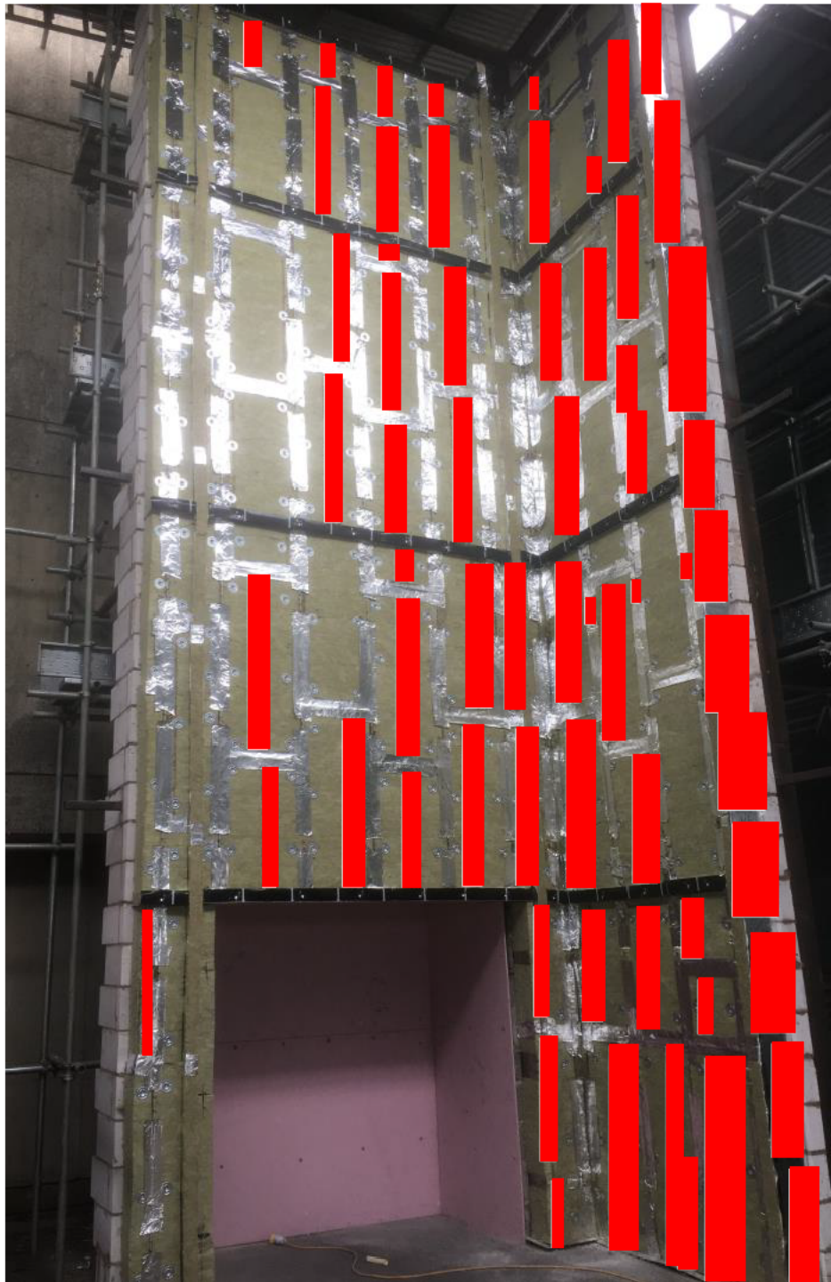
Figure 18 – Insulation and cavity barriers prior to installation of support rails and rainscreen
