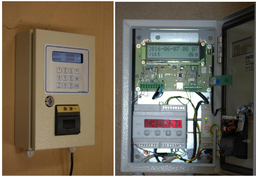
Figure 1 MHS electronics box
