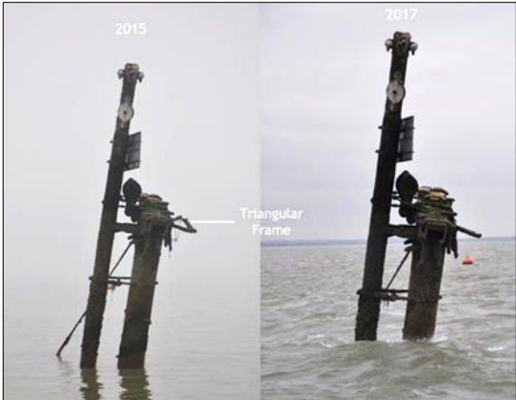
Fig. 23 Fore mast, showing small section of missing frame
