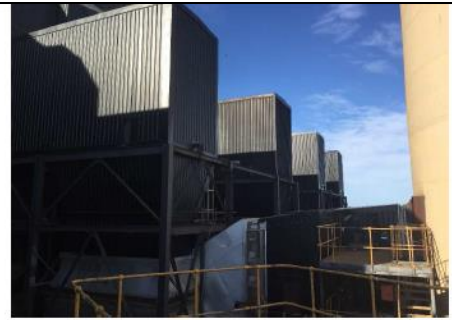
Figure 13: Electrostatic Precipitators (Showing Close Proximity of Unit 1 & 2 ESP Outlets and ID Fan Ductwork to Stack Inlet)
