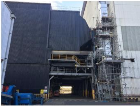
Figure 11: Electrostatic Precipitators (Unit 1 A0 & B0 Fields – Boiler House Visible to Right)
