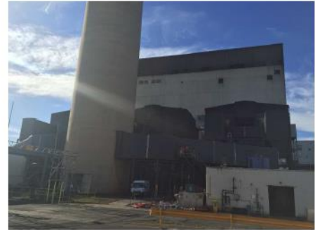
Figure 14: Electrostatic Precipitators (Boiler House Rear, ESPs and Stack Ductwork)
