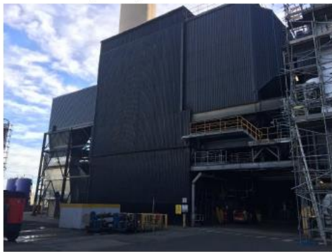
Figure 12: Electrostatic Precipitators (Unit 1 ESP from Boiler House - right, to ID Fan Inlet - left)
