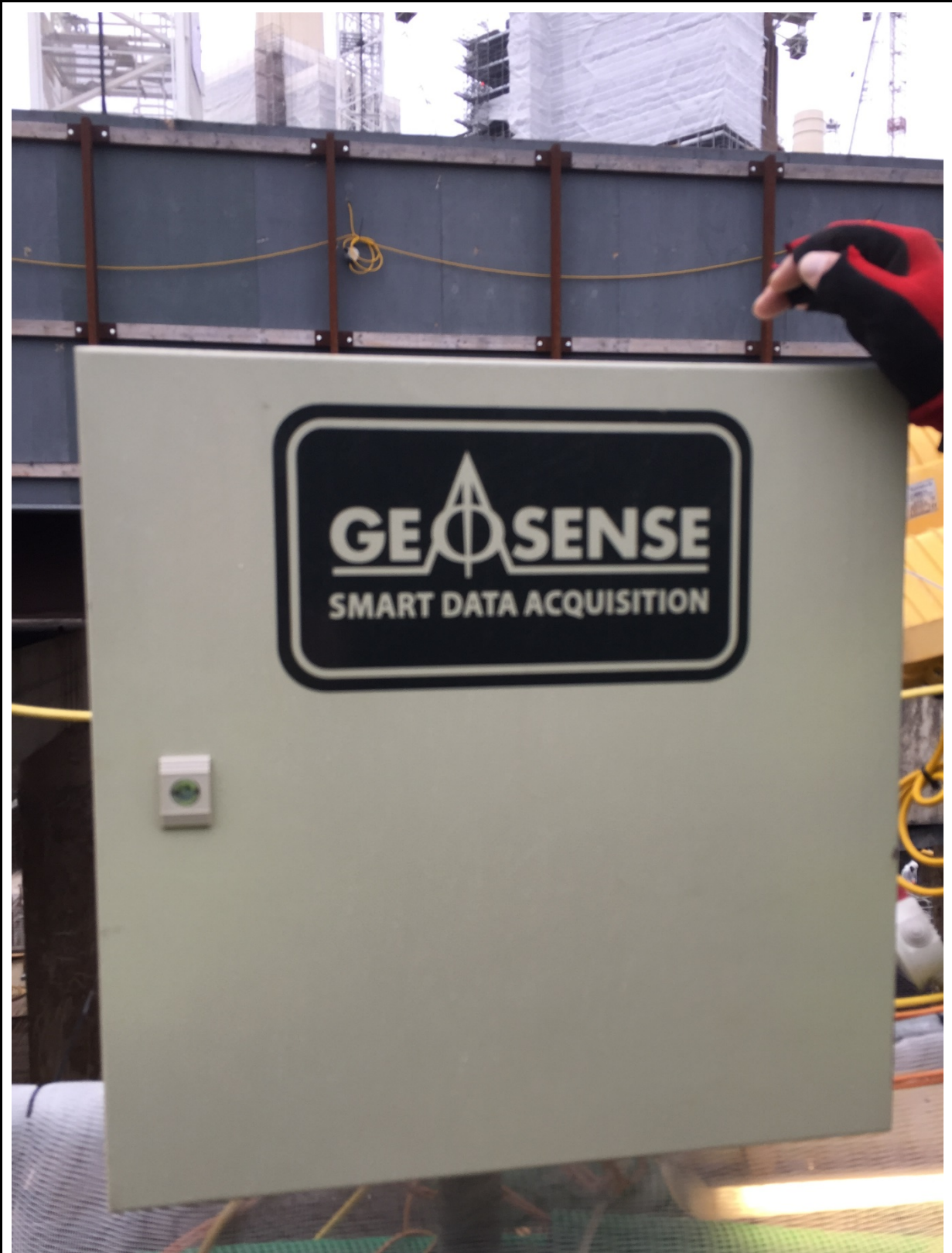
Figure 3: Monitoring ground shift in a massive retaining wall at Battersea Power Station.
