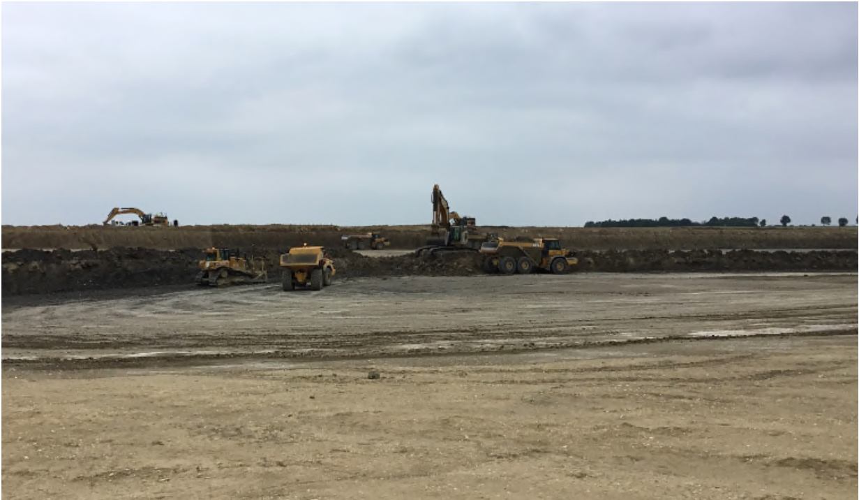
Figure 2: Illustrative example of a typical borrow pit operation (unmitigated) (by permission of Highways England)
