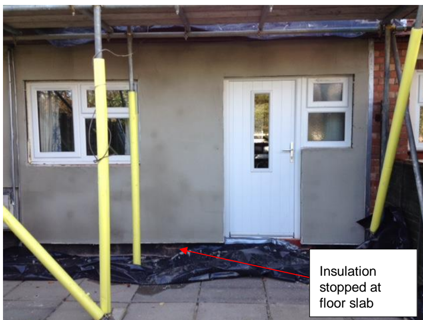
Figure E9 – Insulation stopped above floor slab
