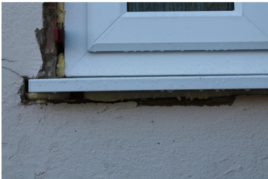
Figure E15- Exposed sub structure and presence of moisture
