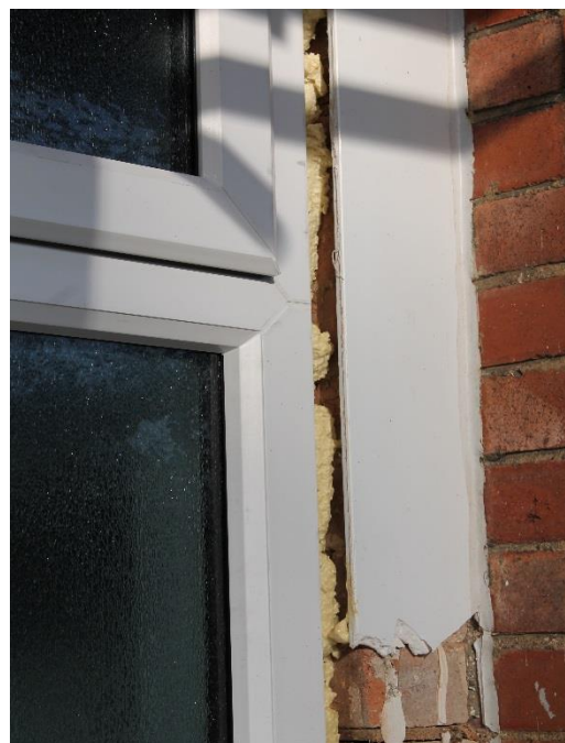
Figure E14 – inconsistent use of foam
