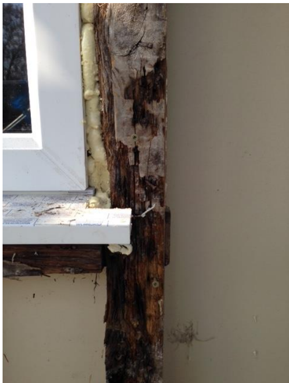
Figure E10 – rotten timber left in place
