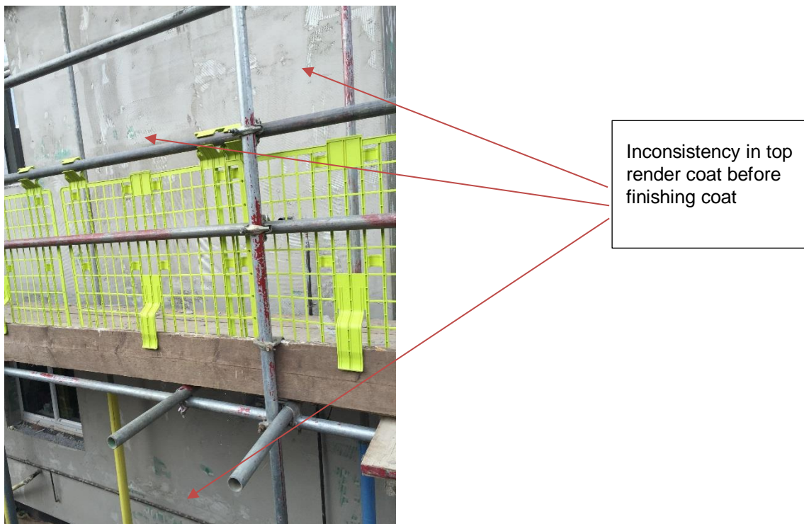
Figure E24. Inconsistency in top render coat before finishing coat
