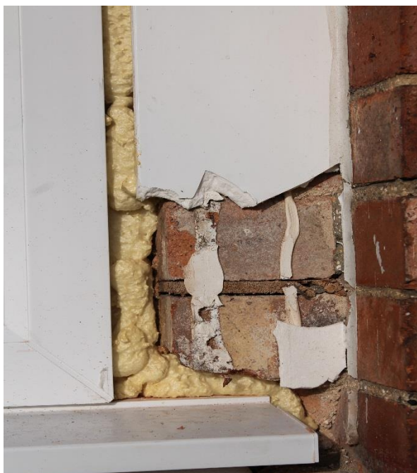
Figure E13 – window packed out with foam
