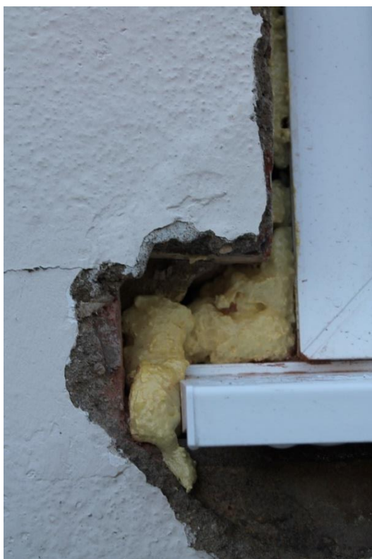
Figure E16 - Exposed sub structure during rain
