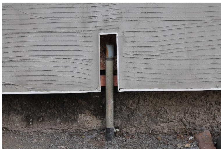
Figure E40 – Poor incoming services detail
