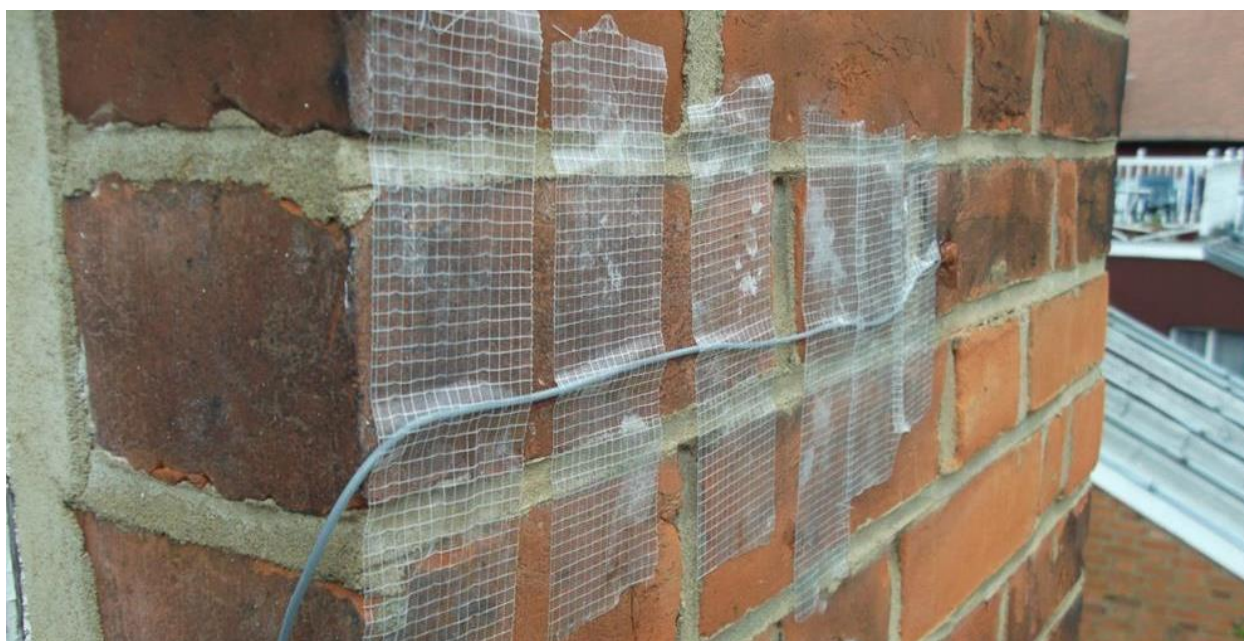
Figure 35 - The external surface sensor
